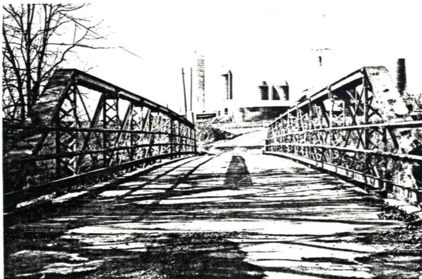
3.9 Dryden, N.Y., Red Mill Road, Fall Creek, 2 span Pratt pony truss, 1887, plank decking.
