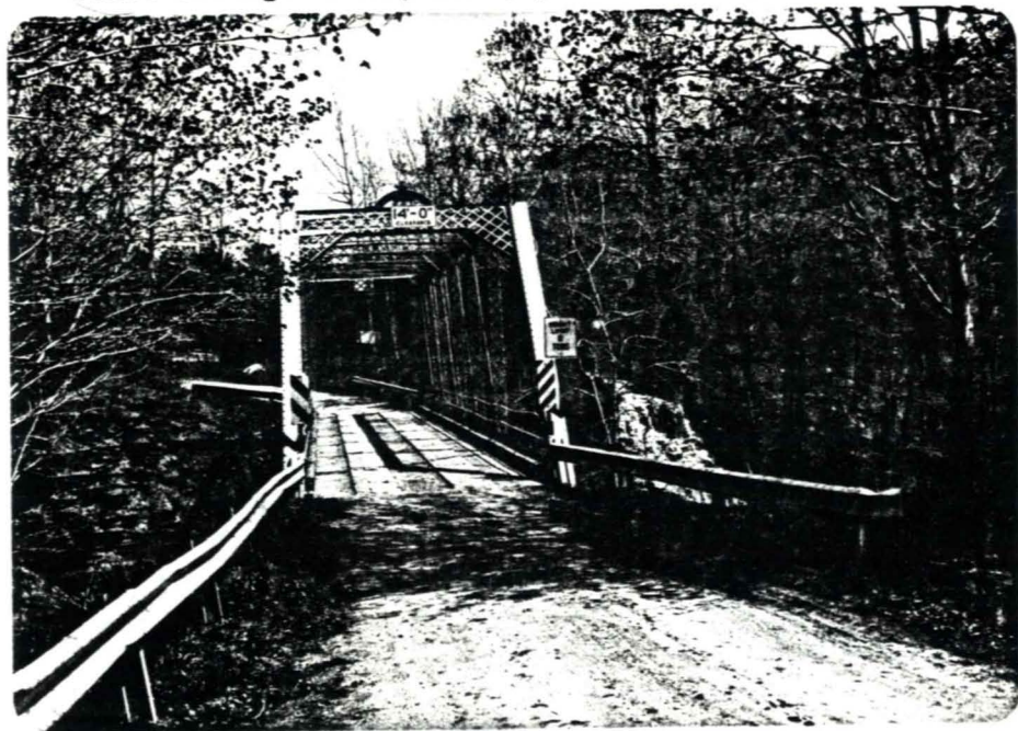
3.67 Worth, N.Y., CR 95, South Sandy Creek, Pratt through truss, 1890, potential NR, approach.
