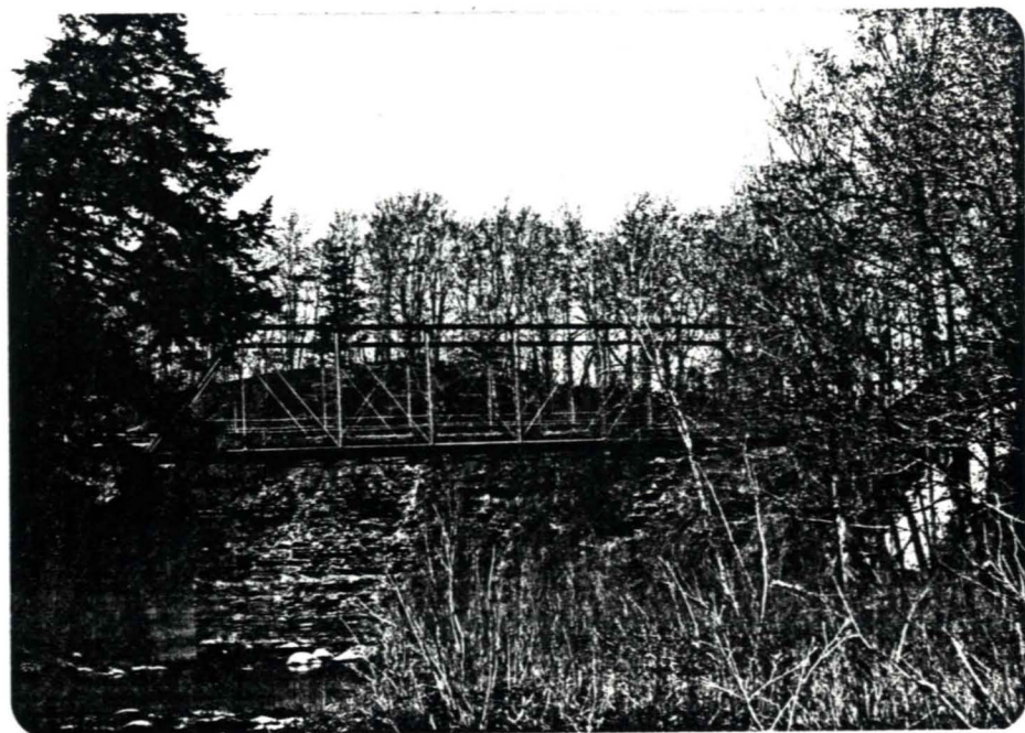
3.66 Worth, N.Y., CR 95, South Sandy Creek, Pratt through truss, 1890, potential NR, elevation.
