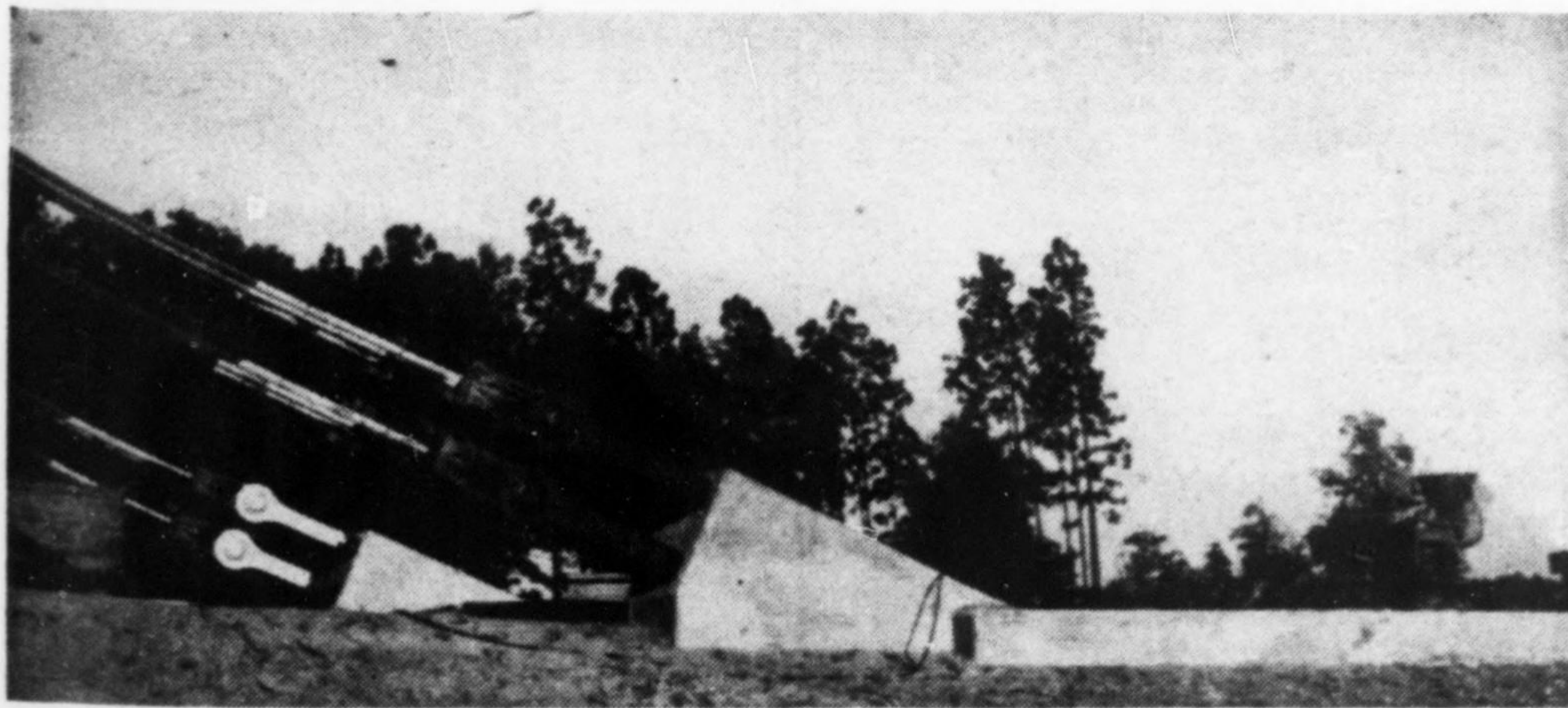
The south anchorage for the main cables is located at roadway level, and consists of a cellular reinforced concrete block. At the anchor blocks, the fitting at the end of each rope of the main cables was attached to two large-diameter steel bolts, which have been left exposed.
