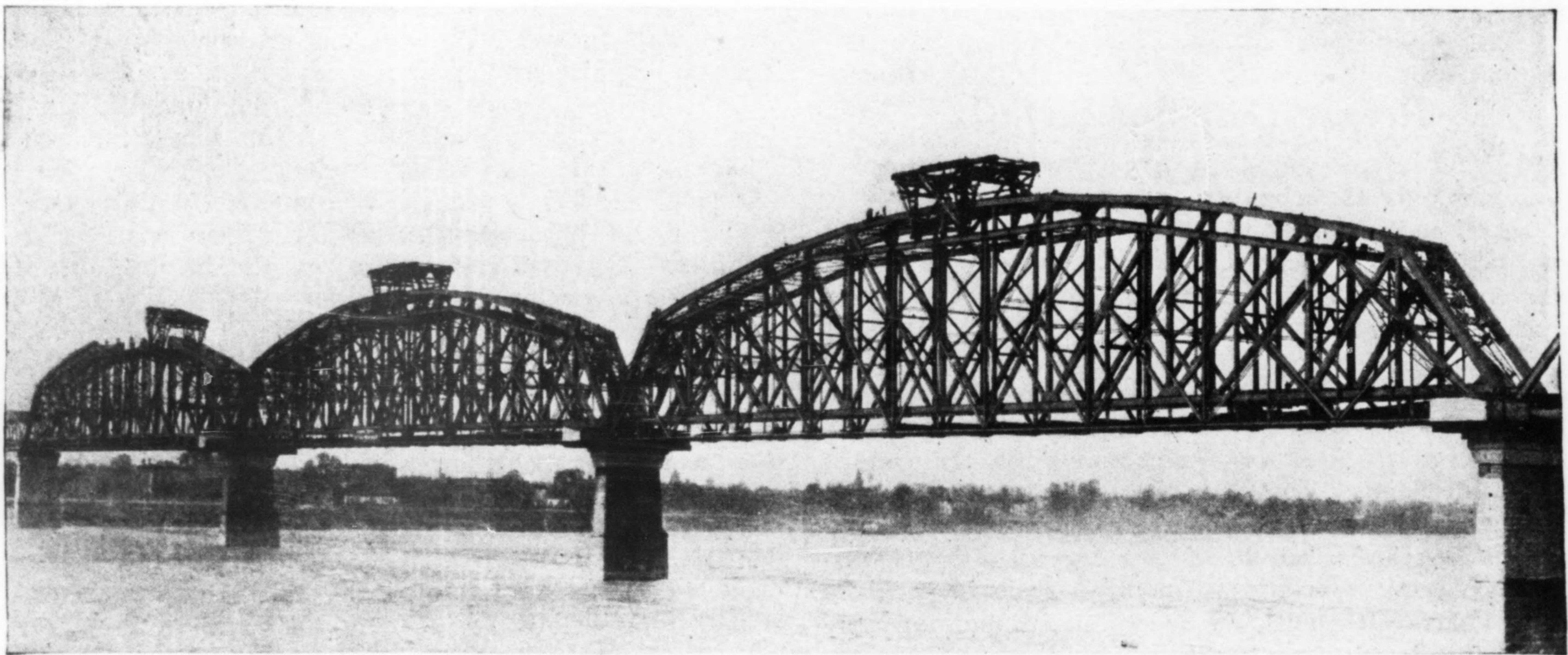
FIG. 1—UTILIZING AN OLD E-30 BRIDGE AS FALSEWORK FOR ERECTING A NEW E-70 STRUCTURE The Ohio River crossing of the Big Four at Louisville, Ky. Travelers are of timber and run on a track on the top chord of the old spans.
