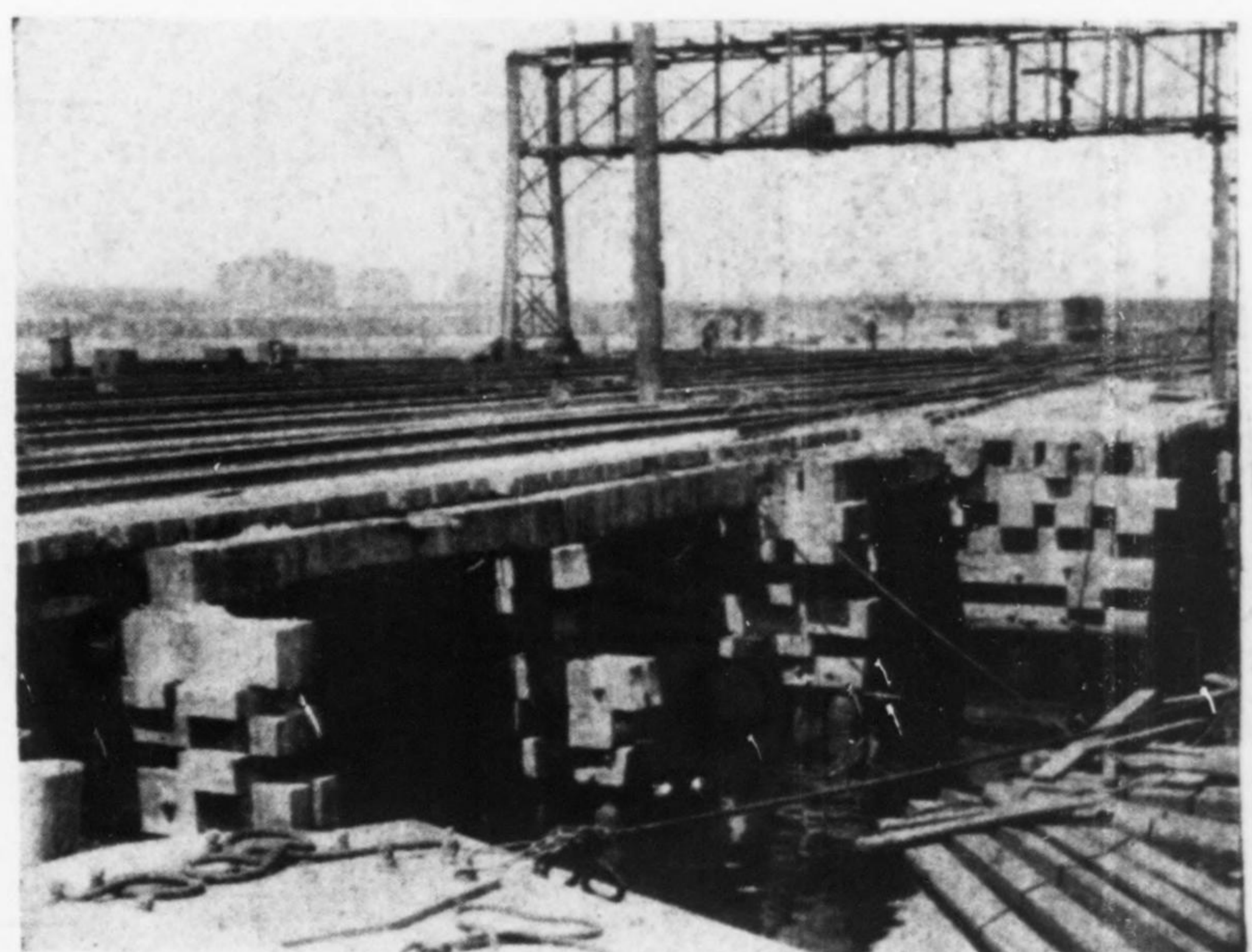
Fig. 7—Maintenance of 65 acres of trestlework in this condition was difficult and expensive
