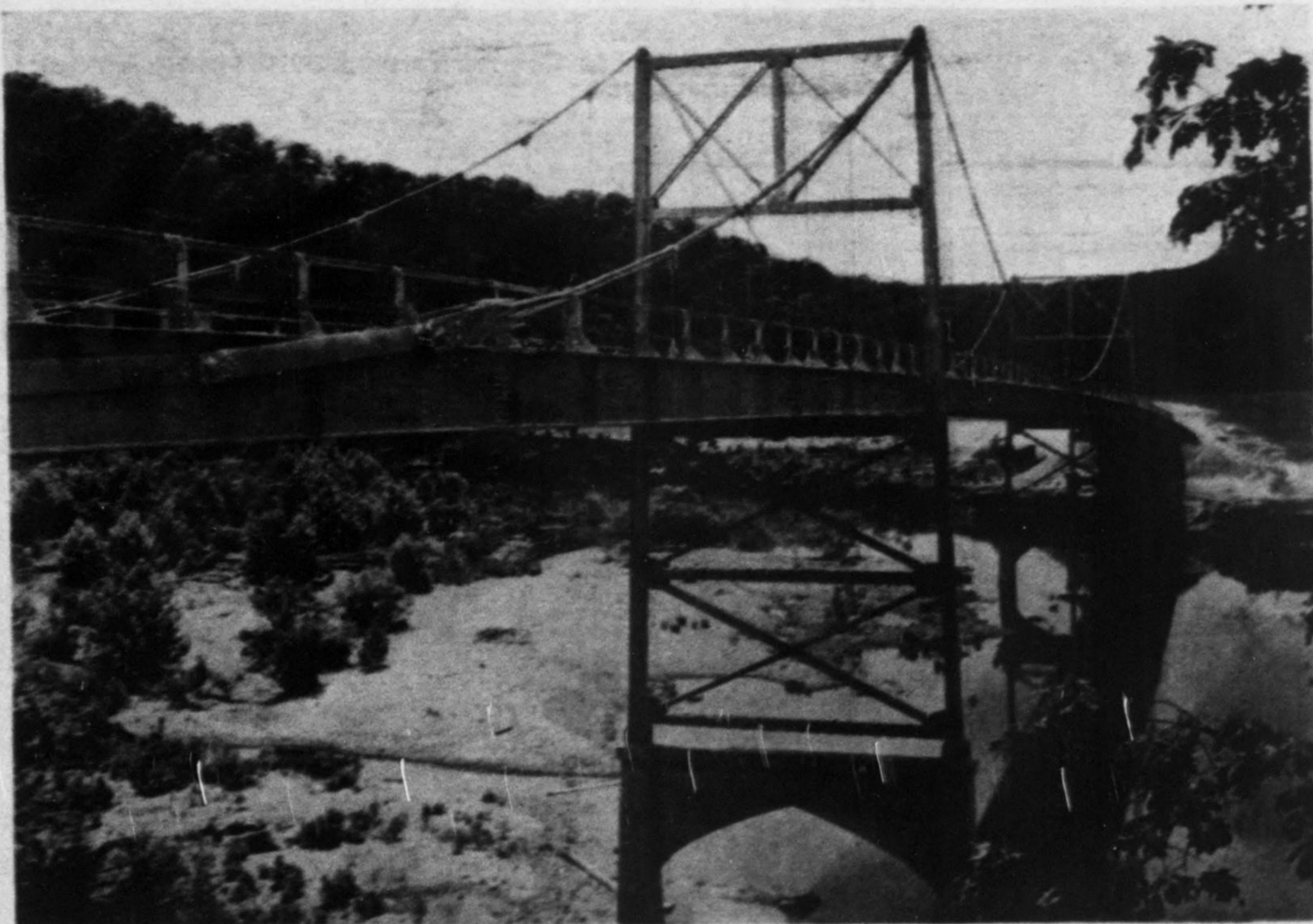
Fig. 1—Short-span self-anchored suspension bridge built by Missouri highway department on a farm-to-market road.
