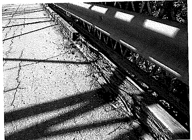
West Side. Showing severe deterioration.
