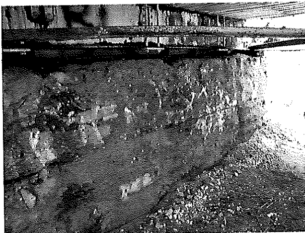
North Side. Showing poor condition.
