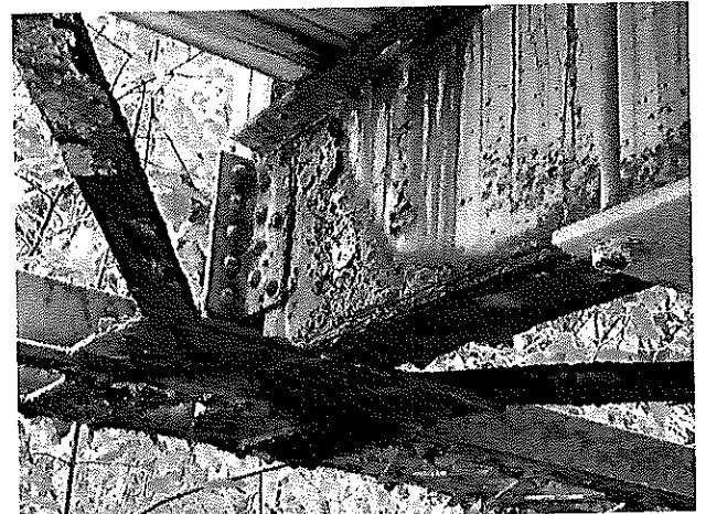
Underside Surface. Showing very severe corrosion.
