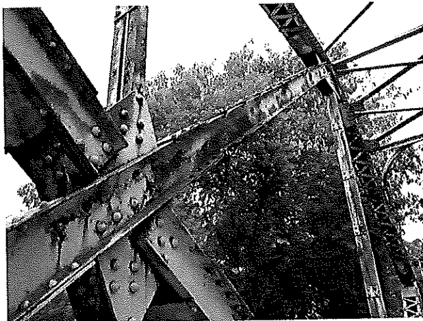
Northwest Side. Showing isolated light deterioration.
