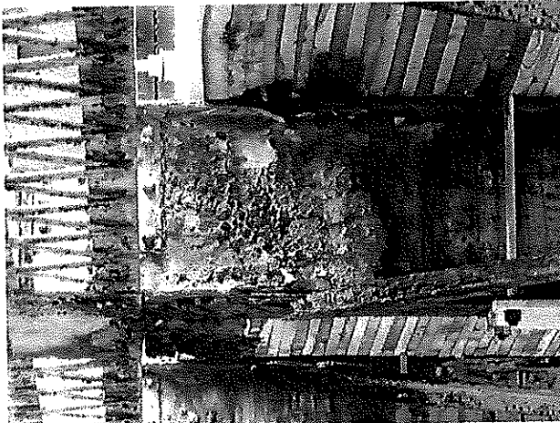
. Showing very severe corrosion.
