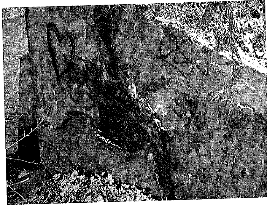
Plate 9 Wing Wall on the East Side of Collingwood Street Bridge on the North Bank
