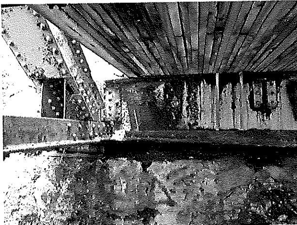
Overall View. Showing severe corrosion.
