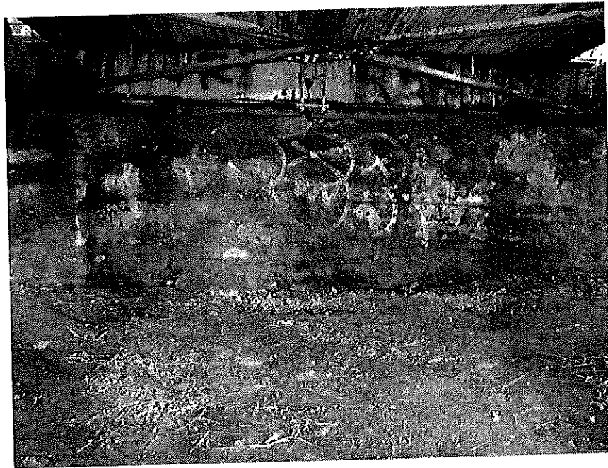
Plate 5 Heavy Corrosion of Supporting Members below the Deck and Condition of the South Abutment
