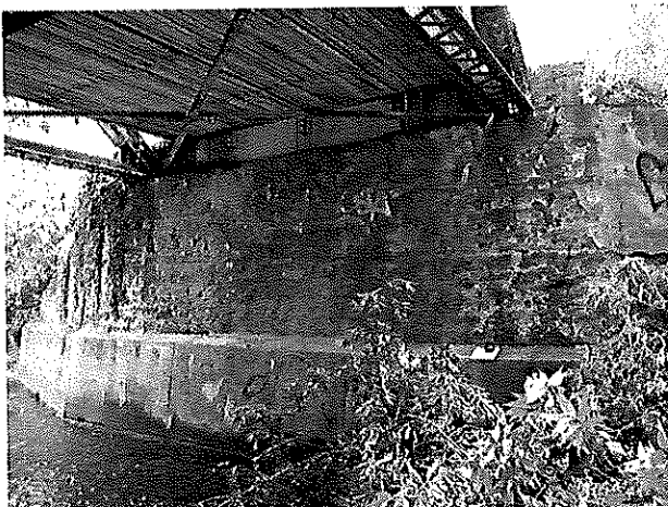
South Side. Showing deterioration.
