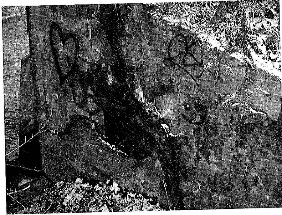
Plate 9 Wing Wall on the East Side of Collingwood Street Bridge on the North Bank
