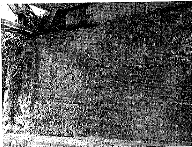
South Side. Showing very severe corrosion.
