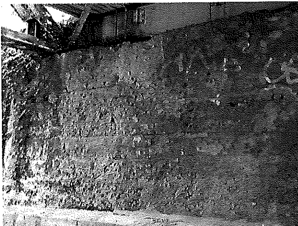
South Side. Showing extensive very severe scaling.
