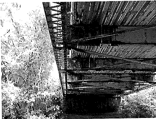
Underside Surface. Showing very severe corrosion.
