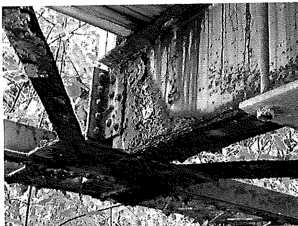
Underside View. Showing very severe corrosion.
