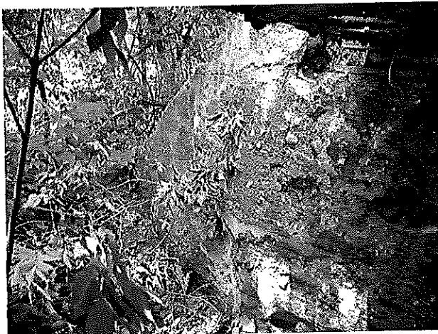
Northwest Side. Showing very severe scaling.
