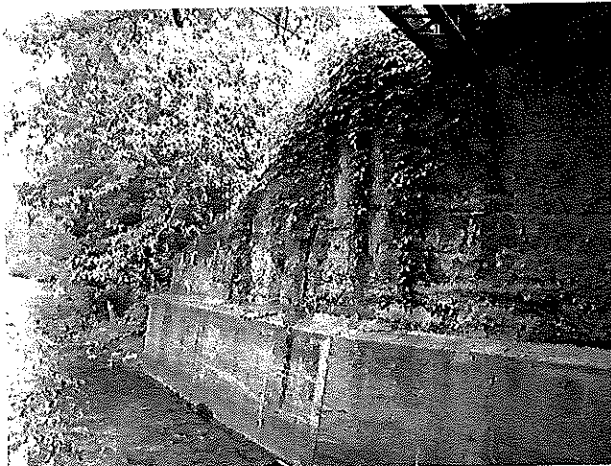
Southeast Side. Showing very severe scaling.
