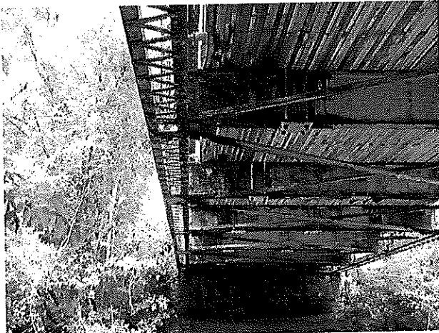
Underside View. Showing very severe condition.
