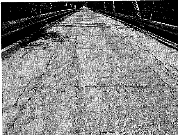
Top Surface. Showing poor condition.
