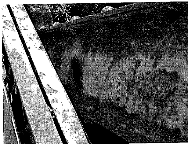
Southwest Side. Showing isolated very severe corrosion.
