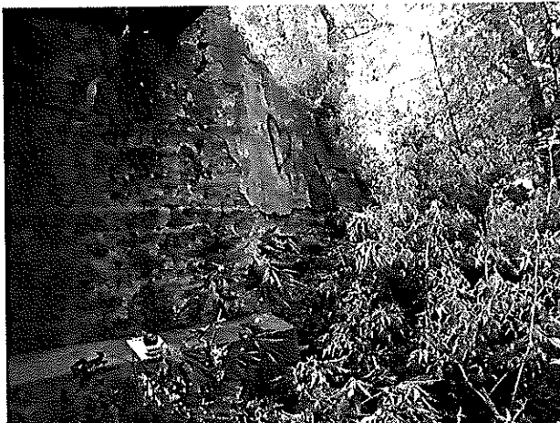
Southwest Side. Showing extensive very severe scaling.
