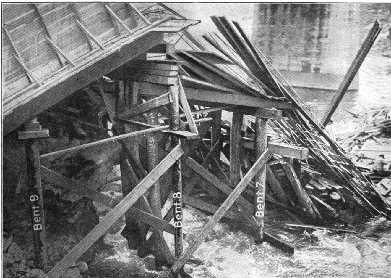
FIG. 4. CLOSE VIEW OF BENTS 7 TO 9 ON WEST SIDE OF POST ST. BRIDGE Pile tops from 9 to 12 in. diameter. Note absence of bolts and presence of shims under half-story round posts
