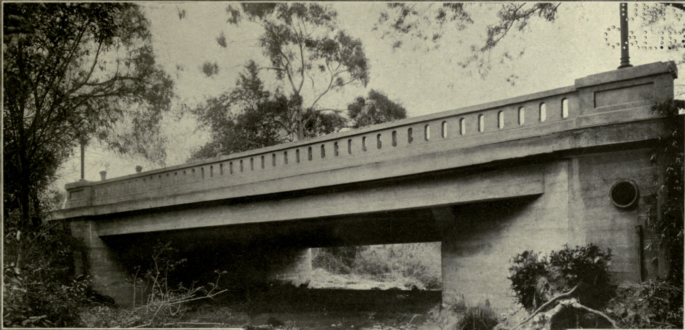
An example of the concrete girder bridge, where a considerable rise of water between low banks was provided for
