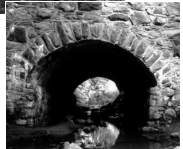
Old Lancaster Pike over Mill Creek Tributary bridge. Arch ring detail showing rubble granite spandrel walls and voussoirs, (State Bridge NC-617).
