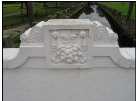
Photo 6-14. Newnan Street Bridge - Molding (No. 724171)
