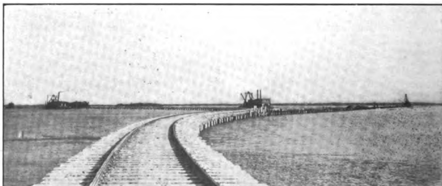
MARL PIT TRESTLE AND DREDGES WHERE MATERIAL FOR PROTECTION OF SLOPES OF EXPOSED EMBANKMENTS IS OBTAINED. KEY WEST EXTENSION, FLORIDA EAST COAST RAILWAY
