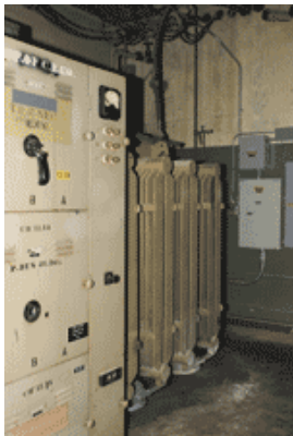
A 12 kV transformer, equipment installed in the original structure in 1943, works with ComEd feed lines coming into the building.
