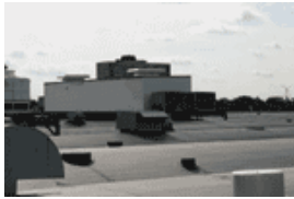
Ford City relies upon rooftop units for each vendor in the mall. Frank and his staff are responsible for the maintenance of each of these units.
