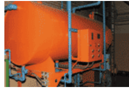
Four Kewanee fire tube boilers were installed in 1976. They supply steam for heating and hot water to the entire mall. Until they were installed, Ford City used the original coal burning equipment installed in 1943.
