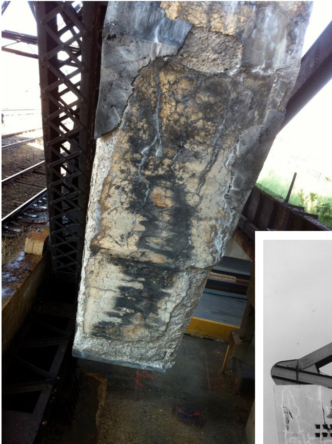
Figure 6 - Condition of the Winged Concrete Counterweight
