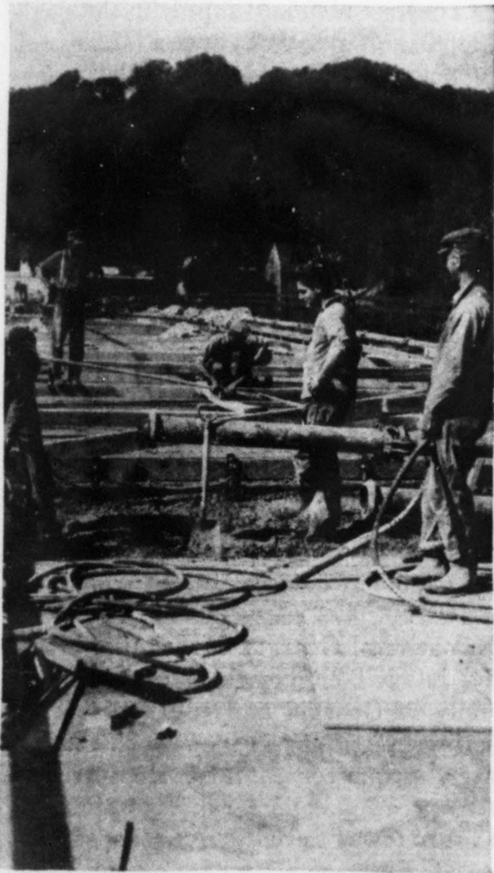
Concrete was delivered at the rate of 20 cu. yds. per hour. It was spread by hand and vibrated in place. The deck was constructed in sections, according to a predetermined sequence.
