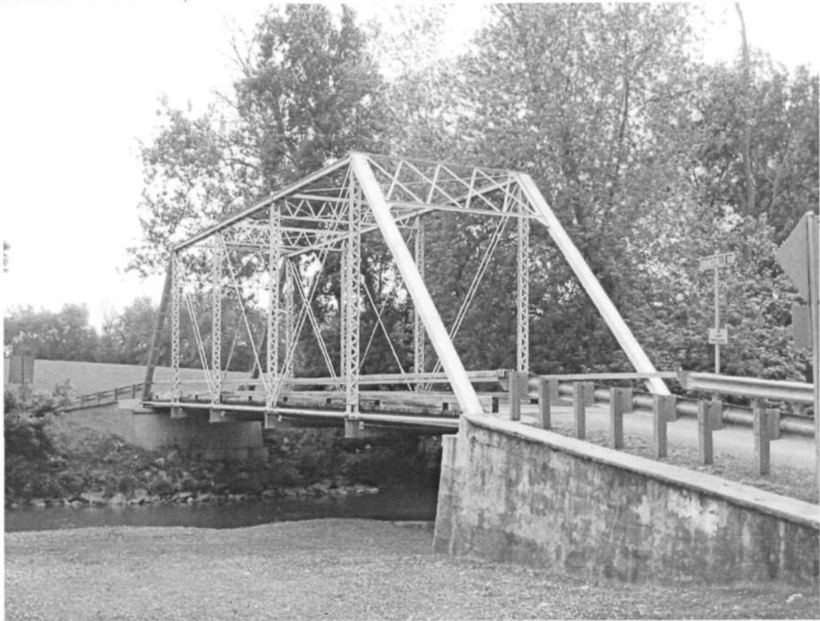
F-8-110 Simpson's Mill Road Bridge Simpson's Mill & Johnsville Roads Jennifer K. Cosham, 10 June 2006
