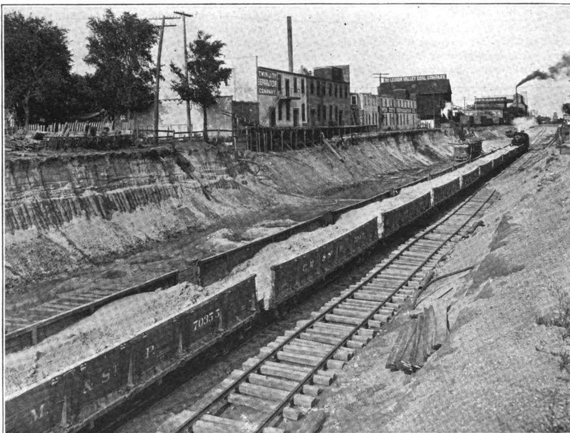
C. M. & St. P. Ry. Track Depression in Minneapolis, Fig. 3—Looking East from Center of Block Between Dupont and Emerson; Shovel in Final Cutting.
