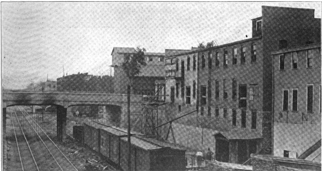
C. M. & St. P. Ry. Track Depression in Minneapolis, Fig. 5—Work at the Twin City Separator Co.
