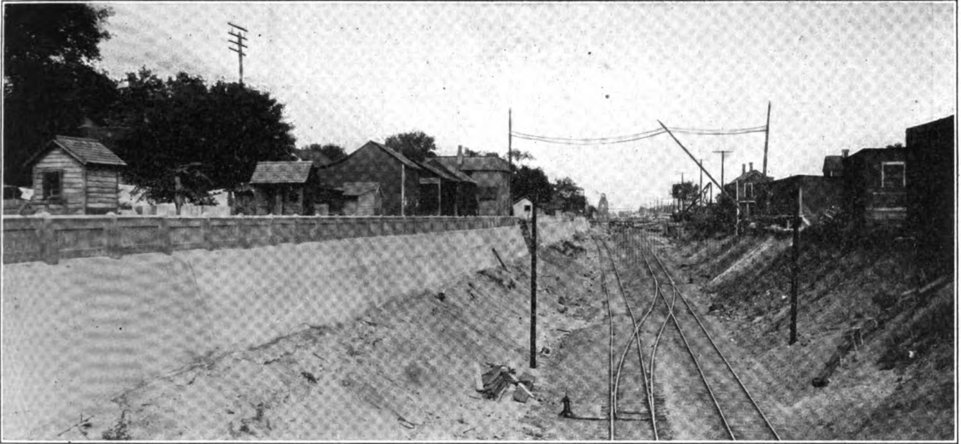
C. M. & St. P. Ry. Track Depression in Minneapolis, Fig. 4—Retaining Wall on North Right of Way Line Between Pleasant and Nicollet.
