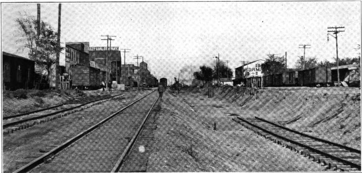
C. M. & St. P. Ry. Track Depression in Minneapolis, Fig. 1—First Cut of Shovel, Looking East from Emerson Ave.
