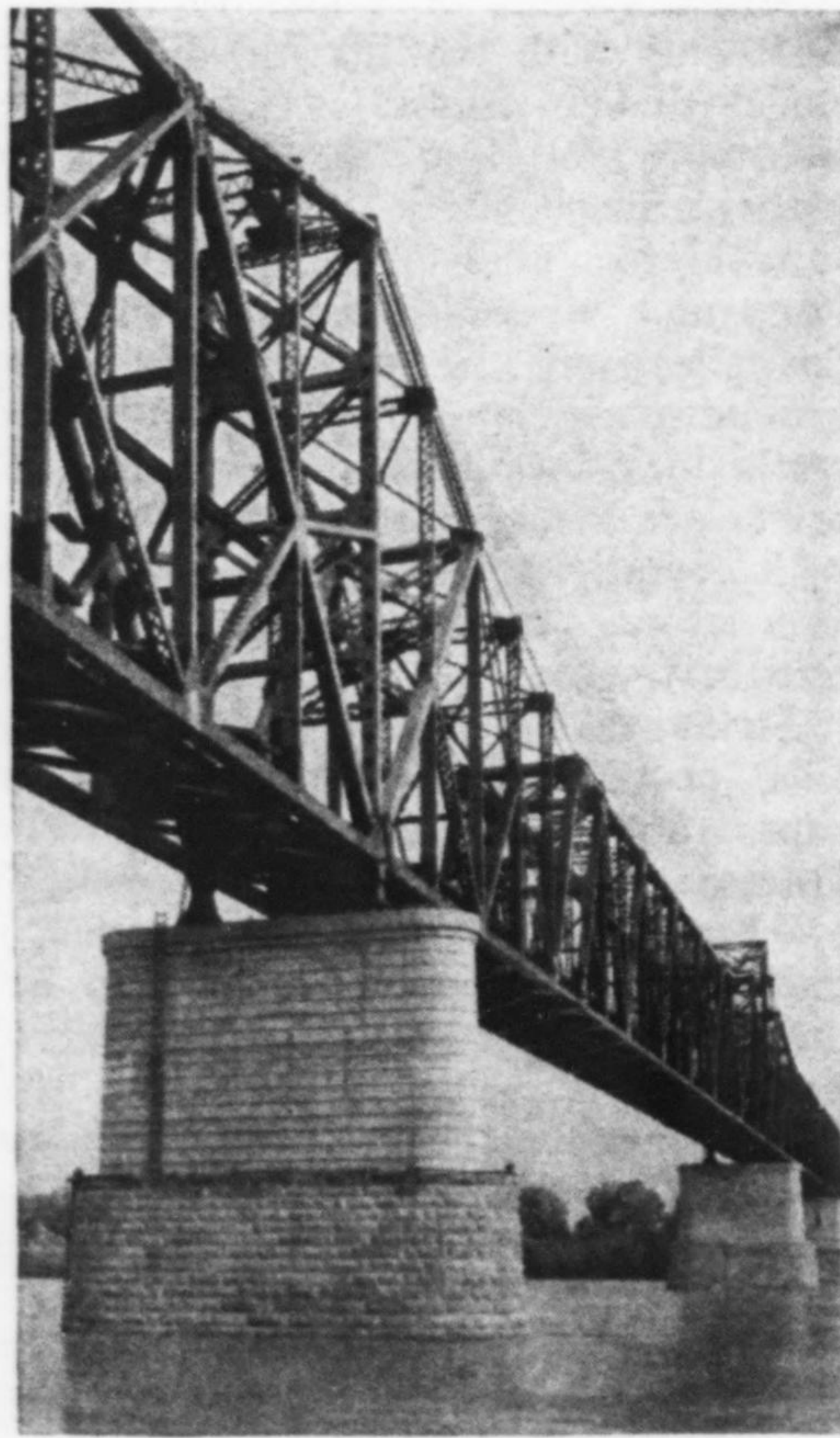
FIG 1—MAIN CANTILEVER span of the new Missouri River crossing of the Wabash Ry. provides a 600 x 45.5 ft. shipping opening.
