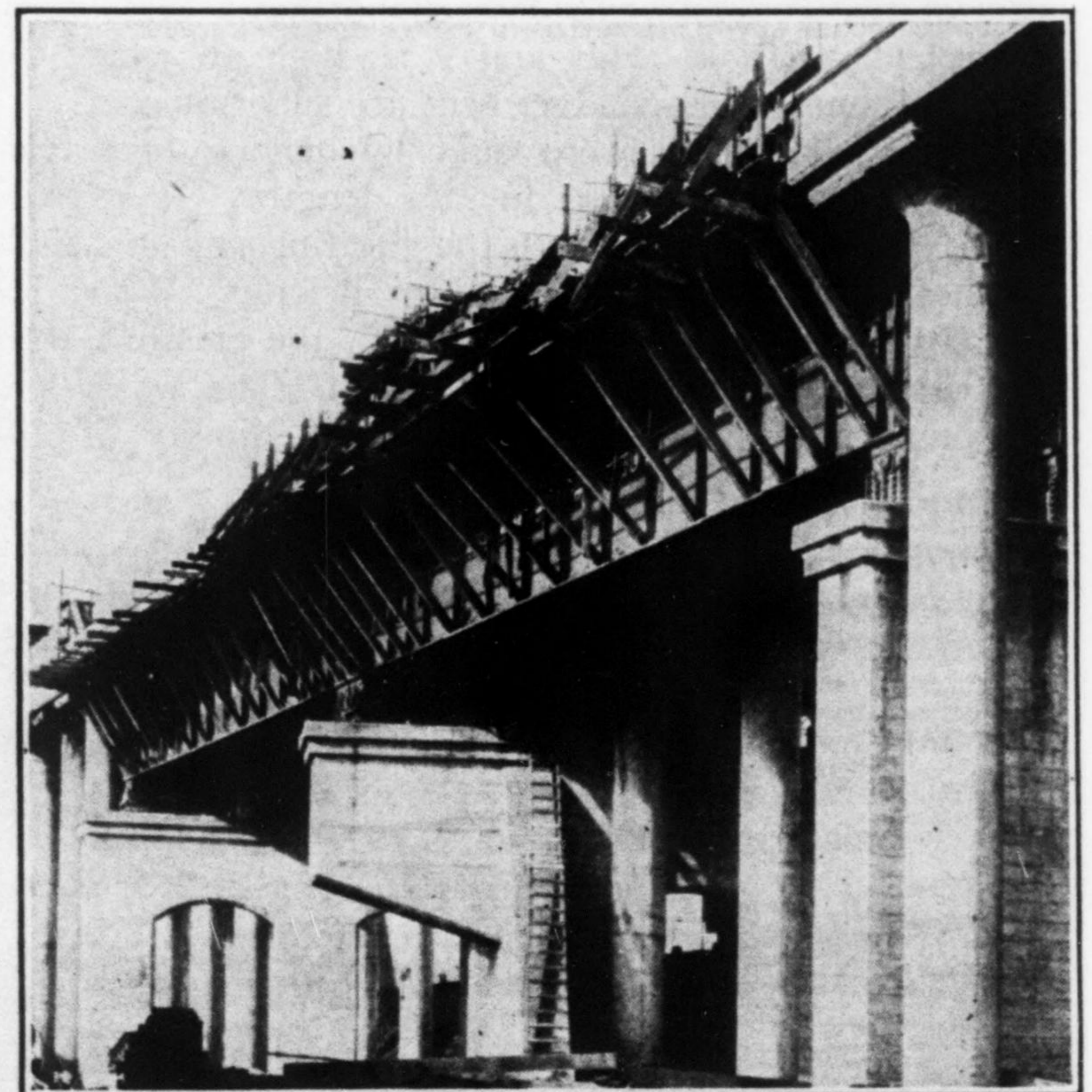
FIG. 5—SLAB FORMWORK ON PLATE GIRDER SPANS Cantilever pier shown built to clear street right-of-way.
