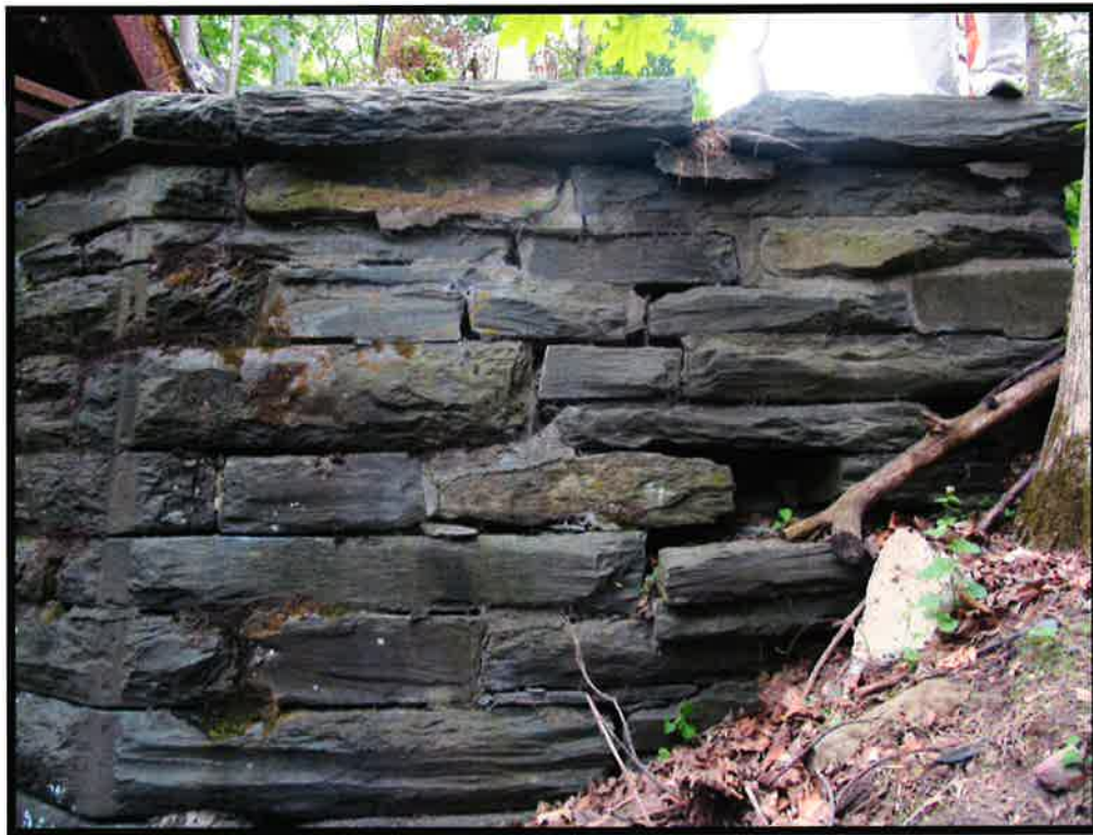
Southerly wing wall, tree should be removed as it is displacing the stonework and stone pushed back to original position
