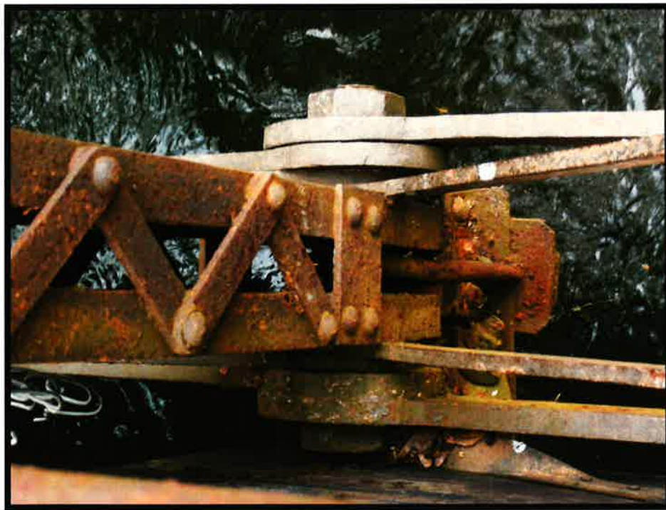
Top view lower chord eyebars, diagonals, vertical post, latticing and floor beam connection
