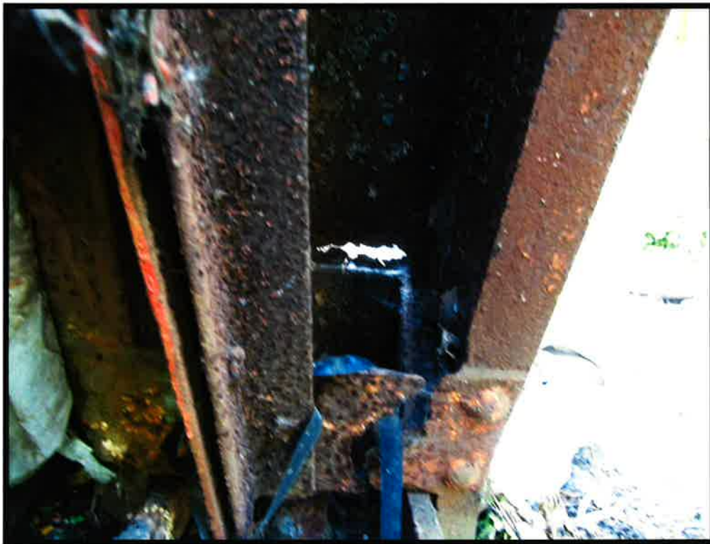
Underside of Southeast bridge seat. Note broken 5 " x 12" plate that should be replaced with new plate farther up the member.
