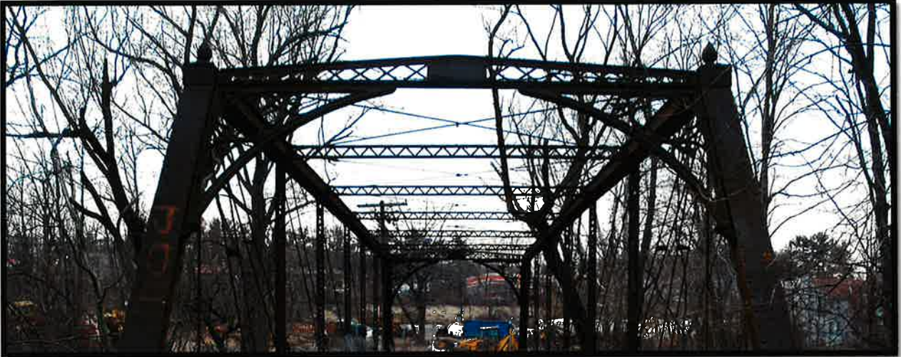
Portal Bracing, wrought iron truss and ornate cast iron tracery (Knee braces)
