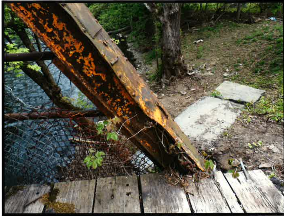
Damaged Inclined End Post, Southwest corner of bridge
