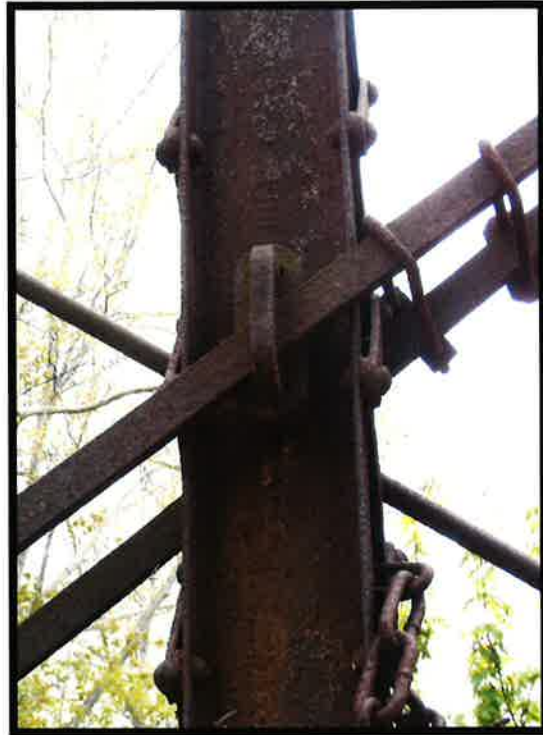
Vertical Posts and brackets for diagonals
