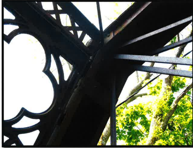
Connection between inclined end post and top chord showing diagonals, vertical and cast iron portal bracing and cross truss.
