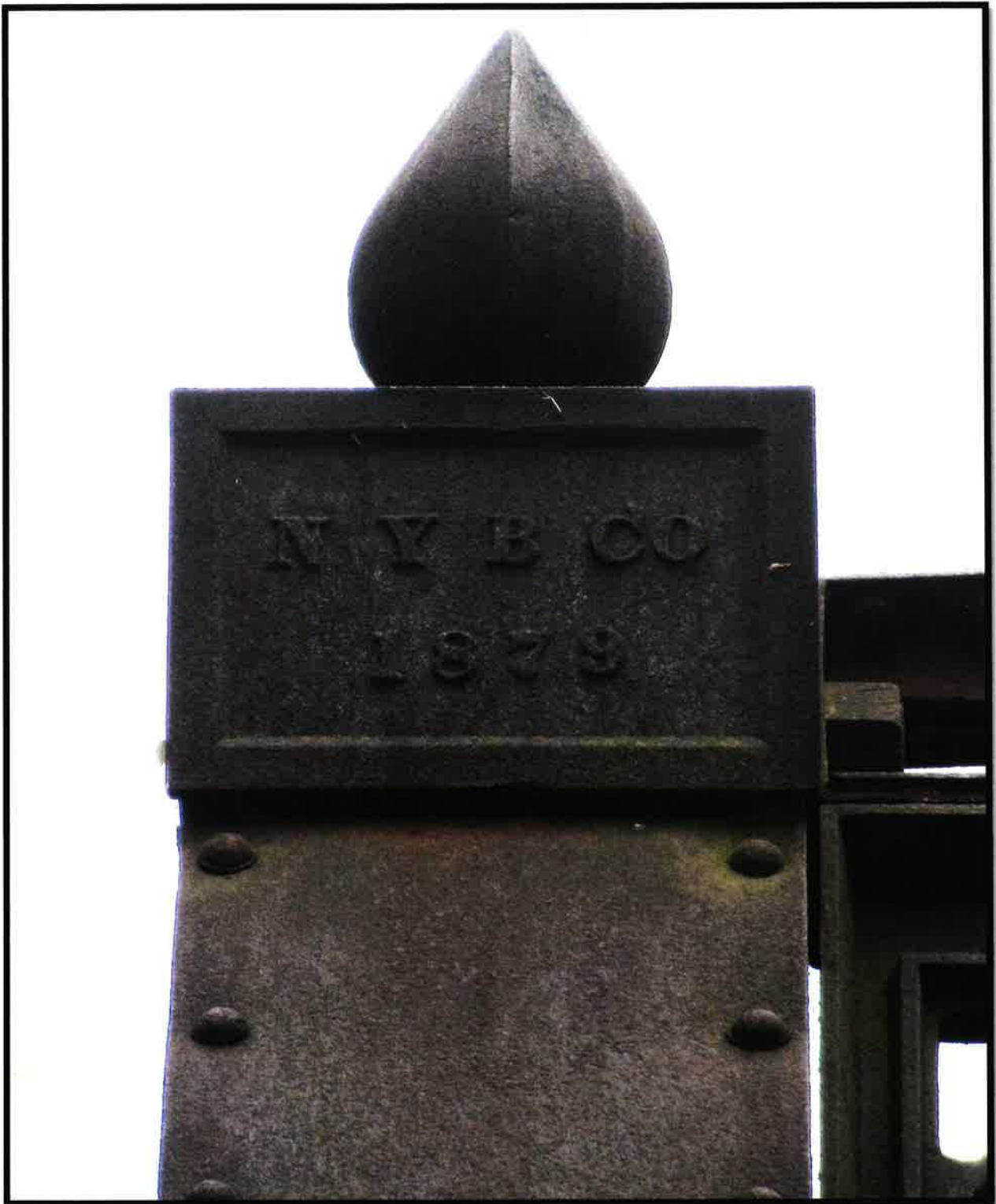
Plaque at top Ends of Truss giving date of construction and Finial.
