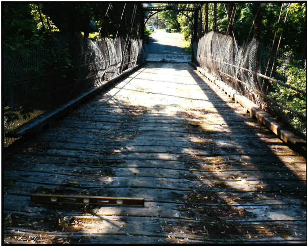
Deck with ruts, with some decay in the rut where water puddles. Depth of rut ~1 1/2".
