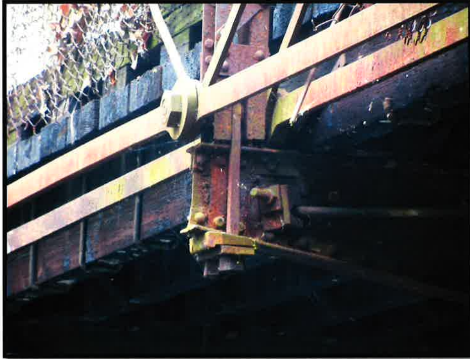
Lower chord eyebars, diagonals, post, diagonal cross bracing, tapered washer and J-bolts to anchor curbing to stringers. L2, L6 (typical) (the web plate at the ends of some of the beams show some section loss at the very ends of the beams).
