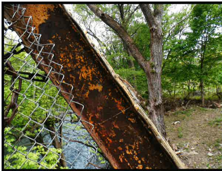
Inclined end post showing rust bulge, pack rust between top plate and channels, lead paint shown.
