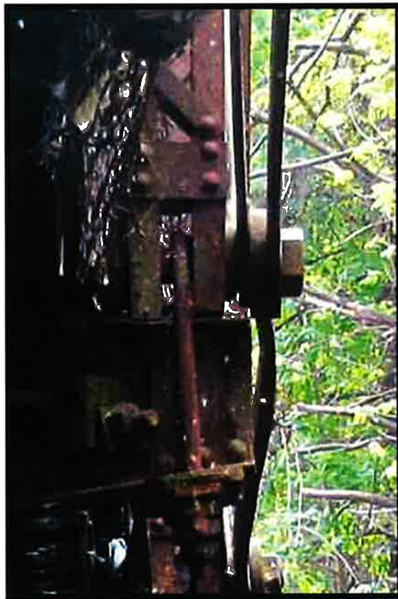
Bottom of posts setting on lower chord pins, and U-Bolts (note bent lower chord member)
