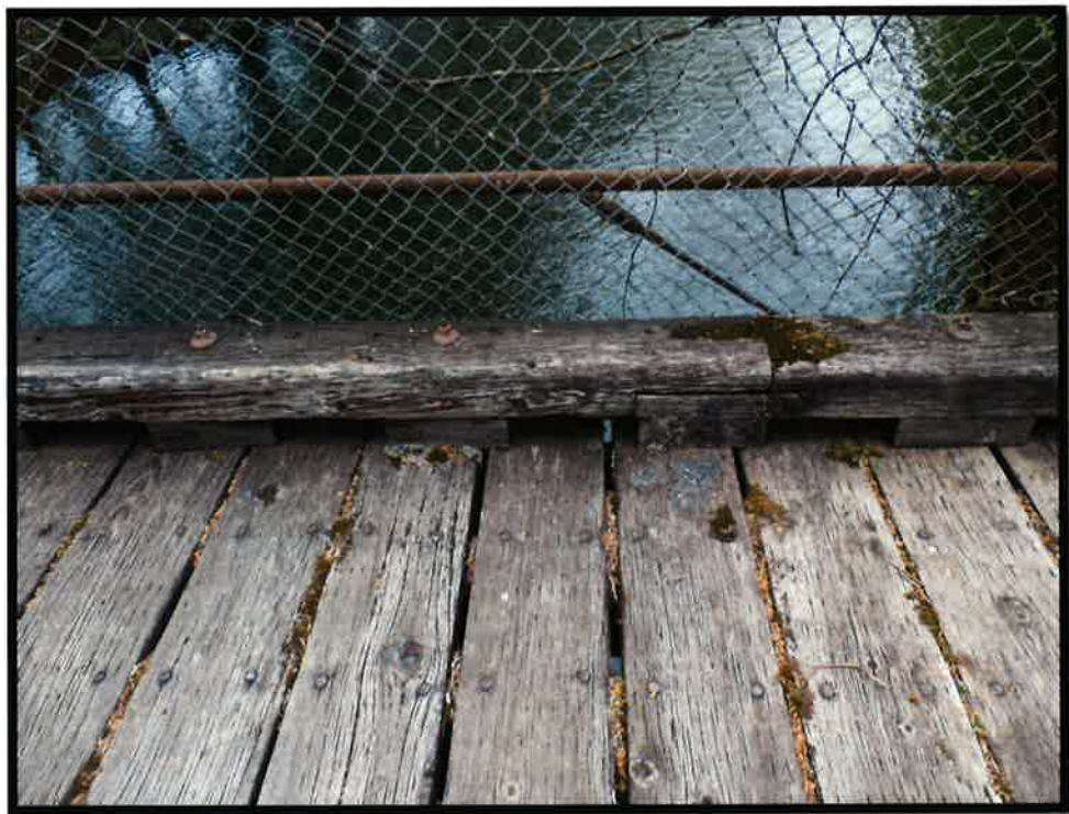
Wooden decking, curb and pipe railing, diagonal, note little decay along edges of decking. Note also organic material collecting in joints. It will be noted later on that this material should be power washed away to minimize further decay in the joint.
