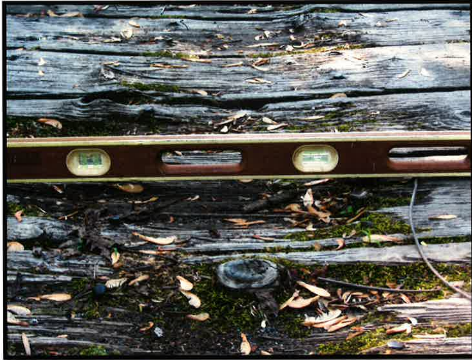
Rut on northerly side of centerline of the bridge showing ~1 ½" depression.
