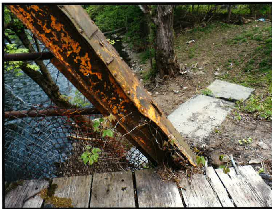
Damaged inclined end post, southwest corner of bridge. Also previously welded plate at top end of image. Some yellow lead paint remains. The lower ~8' of the inclined end posts were painted yellow for visibility purposes
