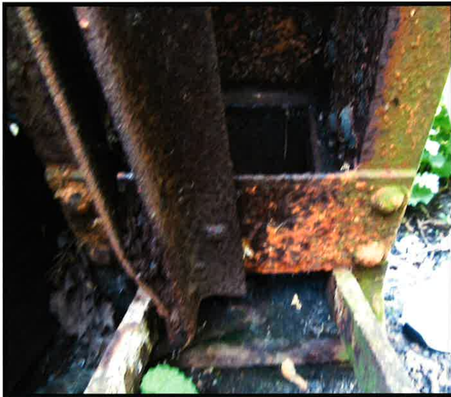
Image under northwest bridge shoe showing bearing surface on cast iron shoe, lower chord links. Note there is no additional bearing plate added to inside face of channels. Pin behind cross plate. Angle on bottom to receive hand railing
