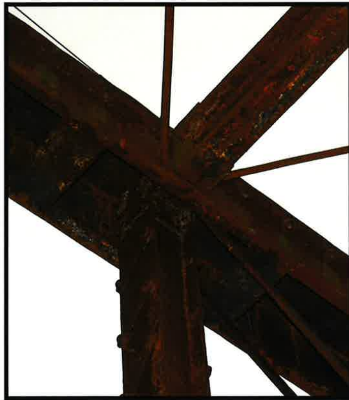
Connection vertical post and top chord showing top chord bracing beam and diagonals.
