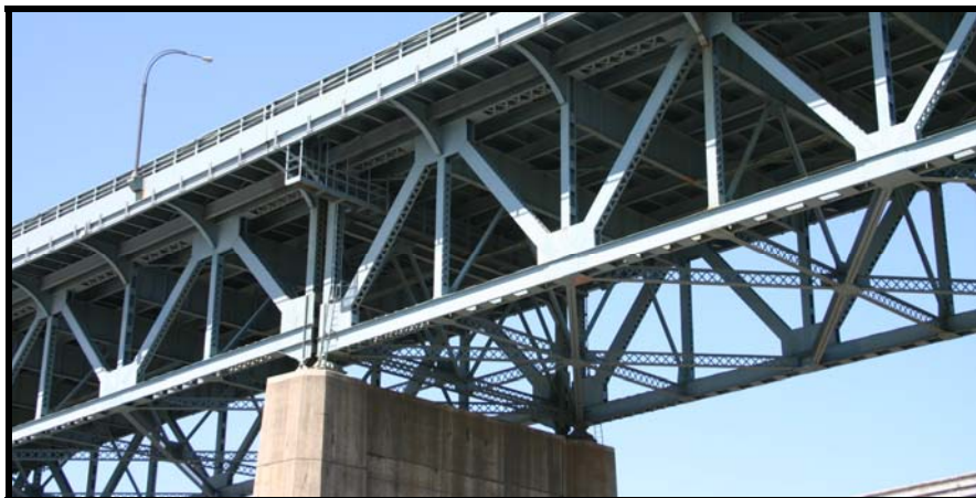
Image 25: Detail showing Warren deck truss of the Kosciuszko Bridge EHT Traceries, May 2006
