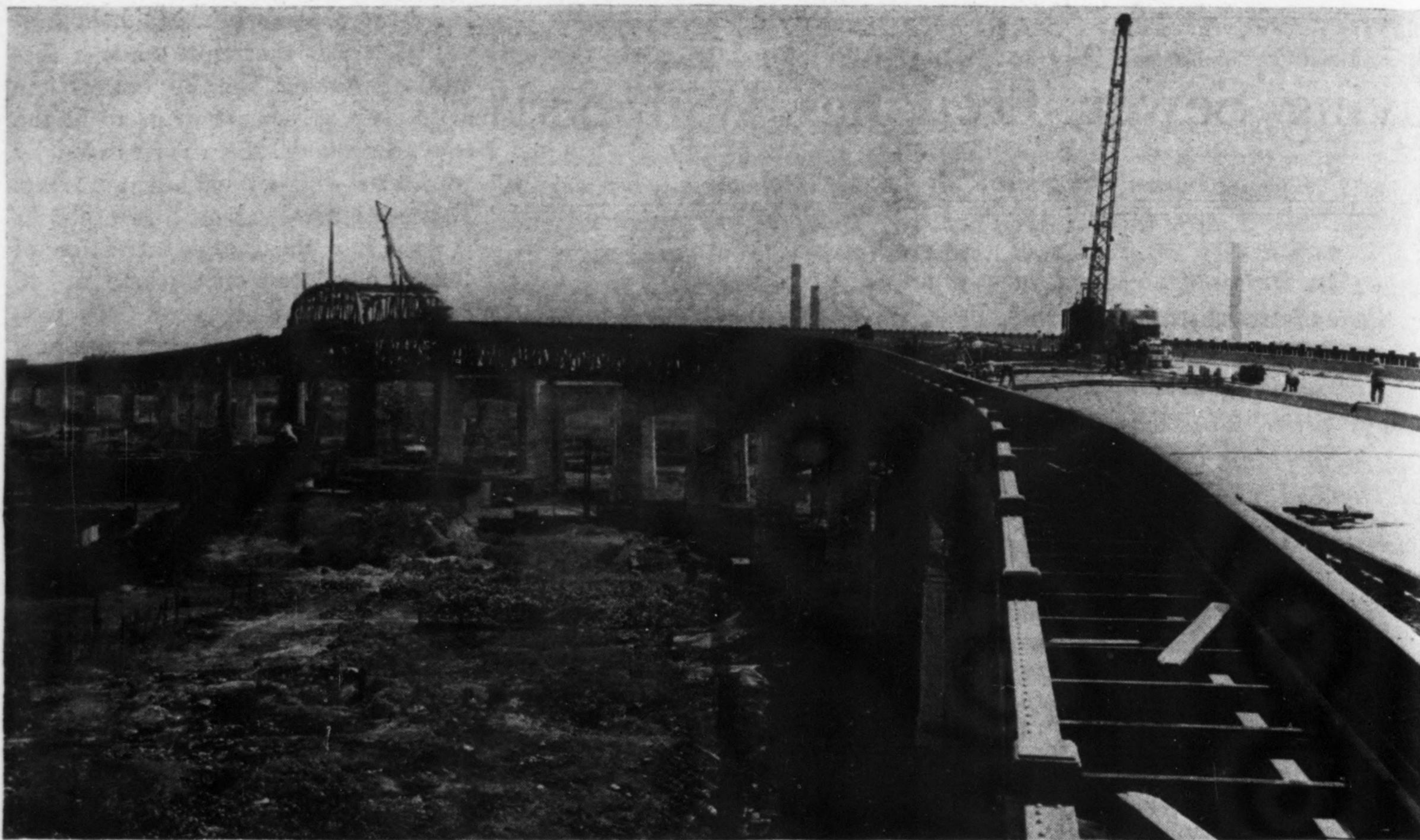
FIG. 1. NEW SIX-LANE DIVIDED HIGHWAY BRIDGE CROSSING BUSY NEWTOWN CREEK AT NEW YORK CITY.
