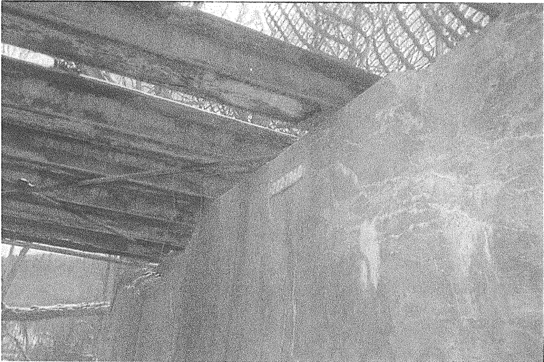
East Abutment looking northerly showing chipping and hairline cracking
