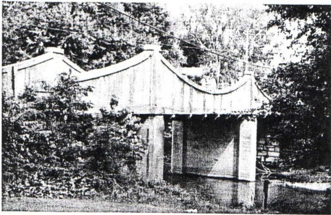
Looking from the side like a concrete suspension bridge, the bridge over Raccoon Creek on old SR 35, adjacent to the Bob Evans Farm in Gallia County, is actually a rare type of concrete cantilever through girder. A construction drawing of a sister bridge in Licking County reveals that the pattern of the reinforcing bars in the girders resembles a steel truss, radiating out from the tops of the tower-like profiles.
