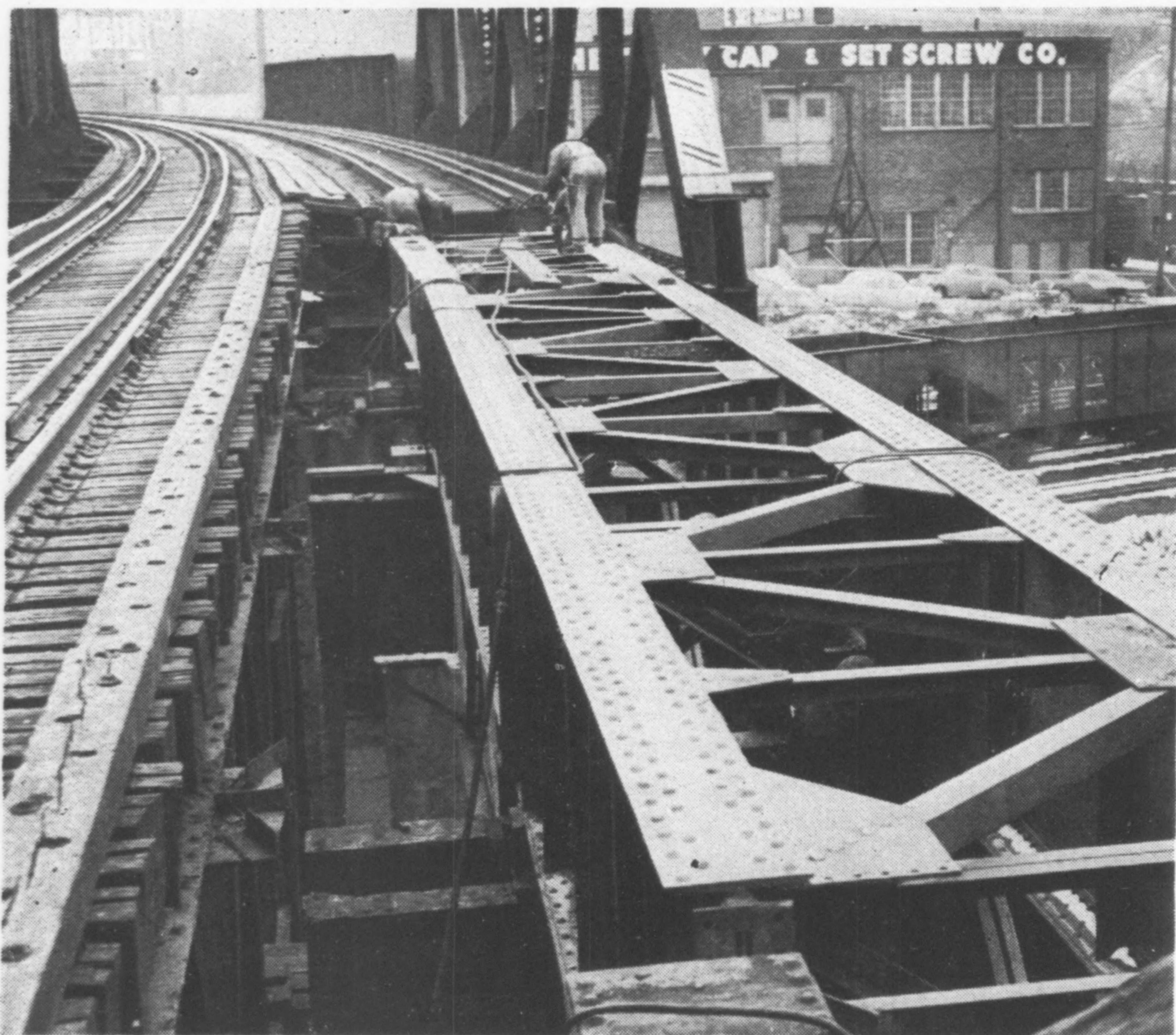
ONE TRACK carries traffic in both directions, while new floor system is installed on other to meet new span.
