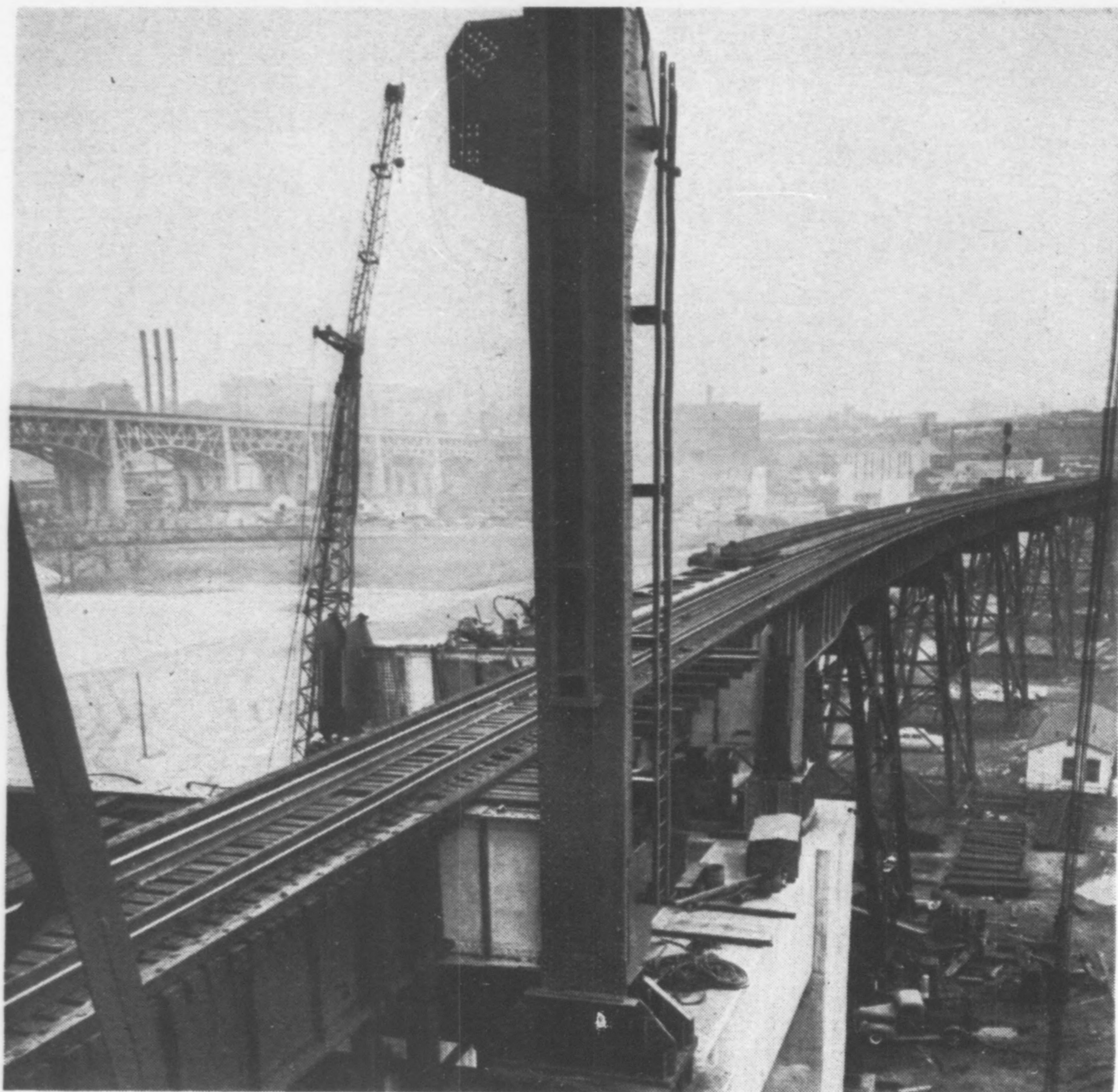
WHILE TRACK WORK goes ahead and new trestle supports go in, steel begins to rise (center) for lift tower.
