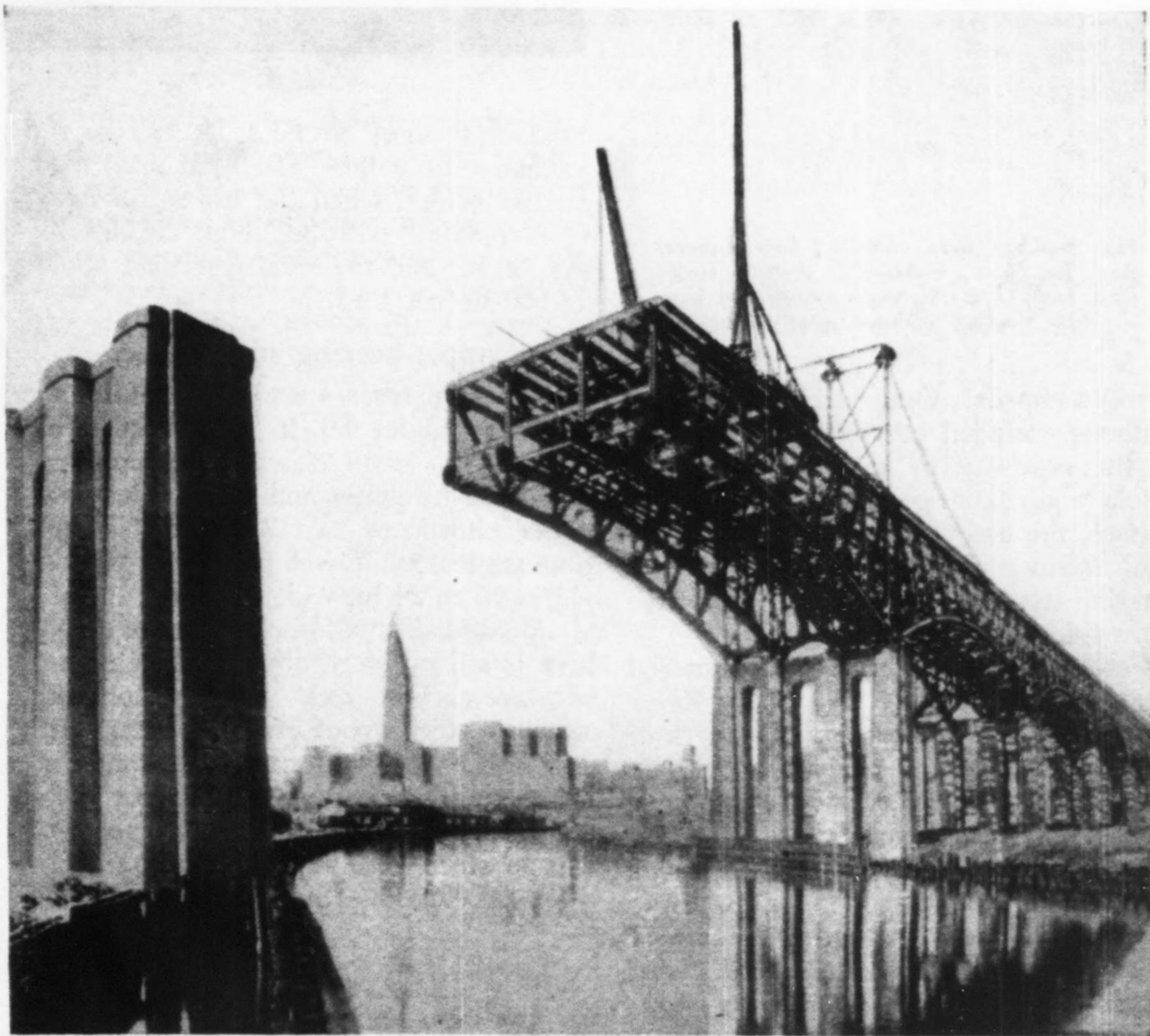
Fig. 2—Erecting the 299-ft. span over the Cuyahoga River. All trusses are cantilevers carrying suspended portions.
