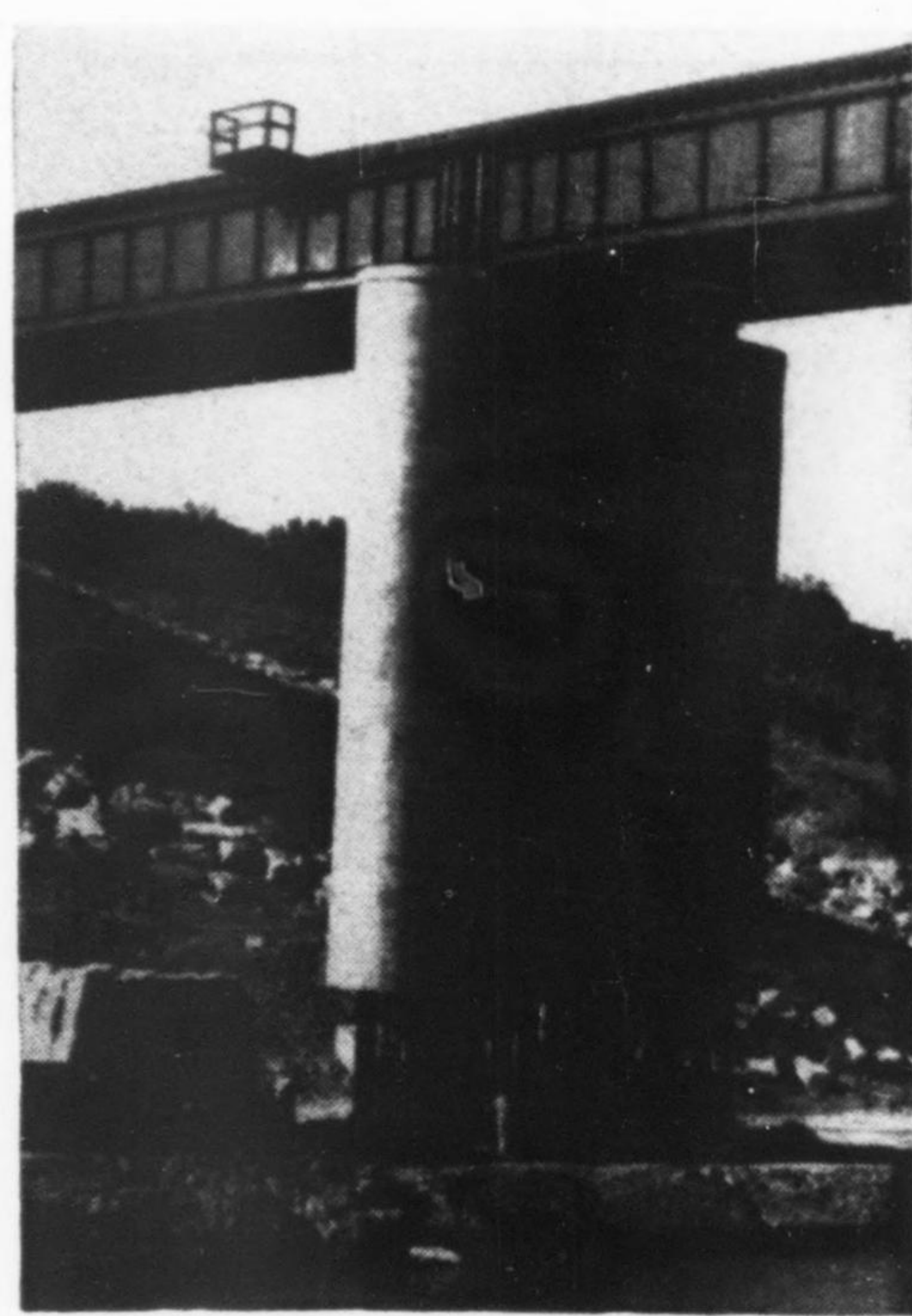
Fig. 10. Excavation below the ground line after the upper section was completed temporarily exposed the bearing piles of Pier 3, while under full load.
