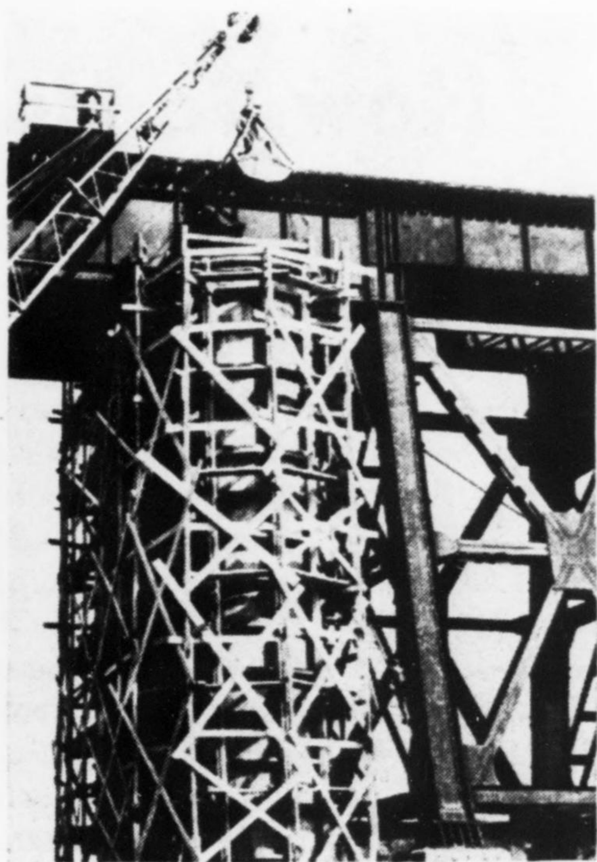
Fig. 9. Graded stone was placed in the pier encasement form by clamshell bucket and grout intruded to complete the pier.
