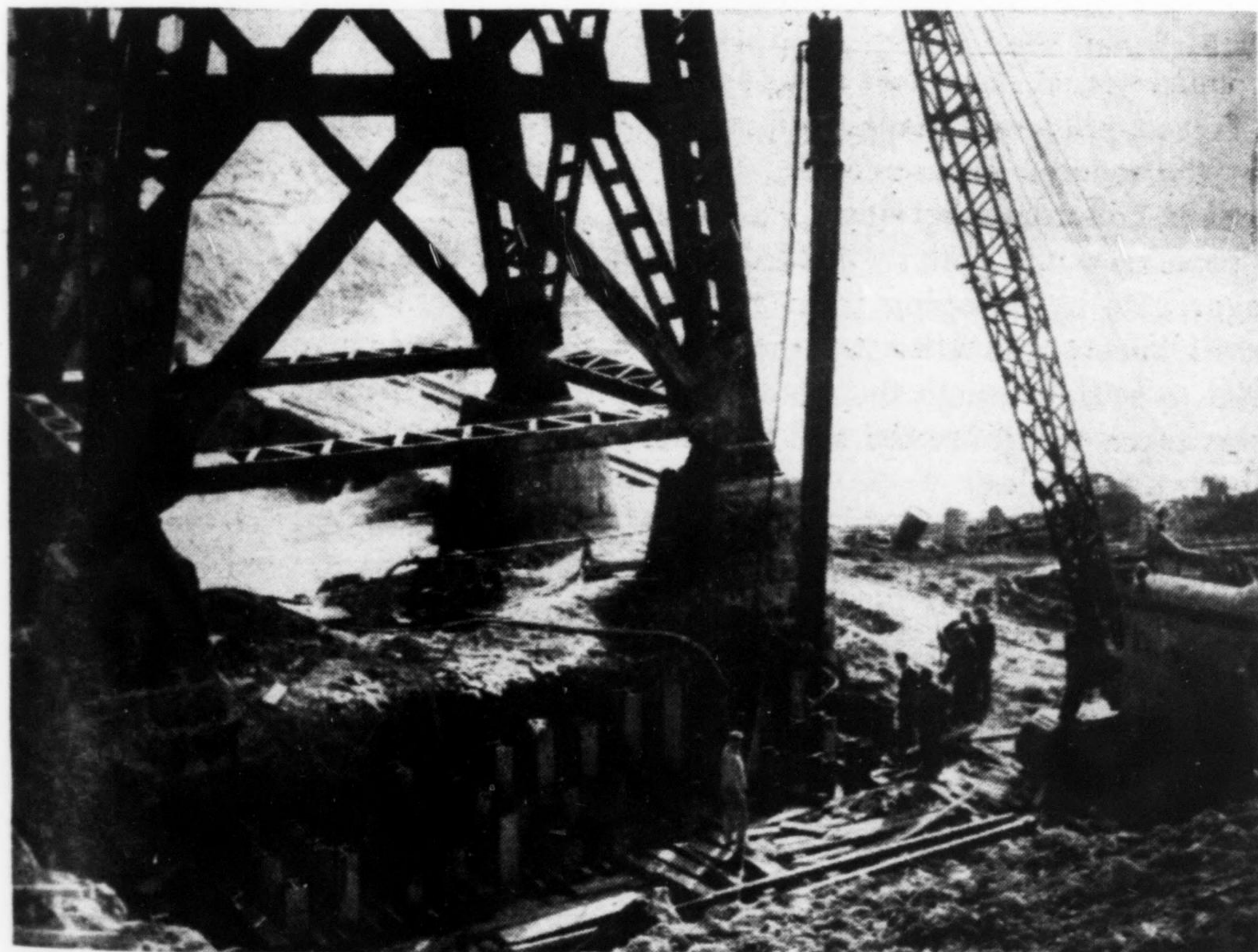
Fig. 6. Pier 3 was constructed immediately adjacent to existing footings by driving H-piles to bearing materials and extending them upward to near the bridge
