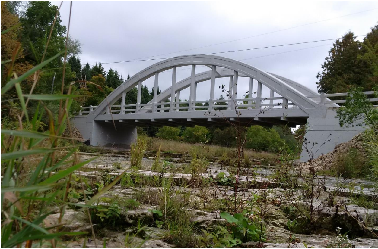
Figure 7: Bridge 9-N after rehabilitations in 2016, a representative example of a concrete bowstring arch bridge Designated under Part IV of the Ontario Heritage Act (CIMA+ email communication 5 December 2018).
