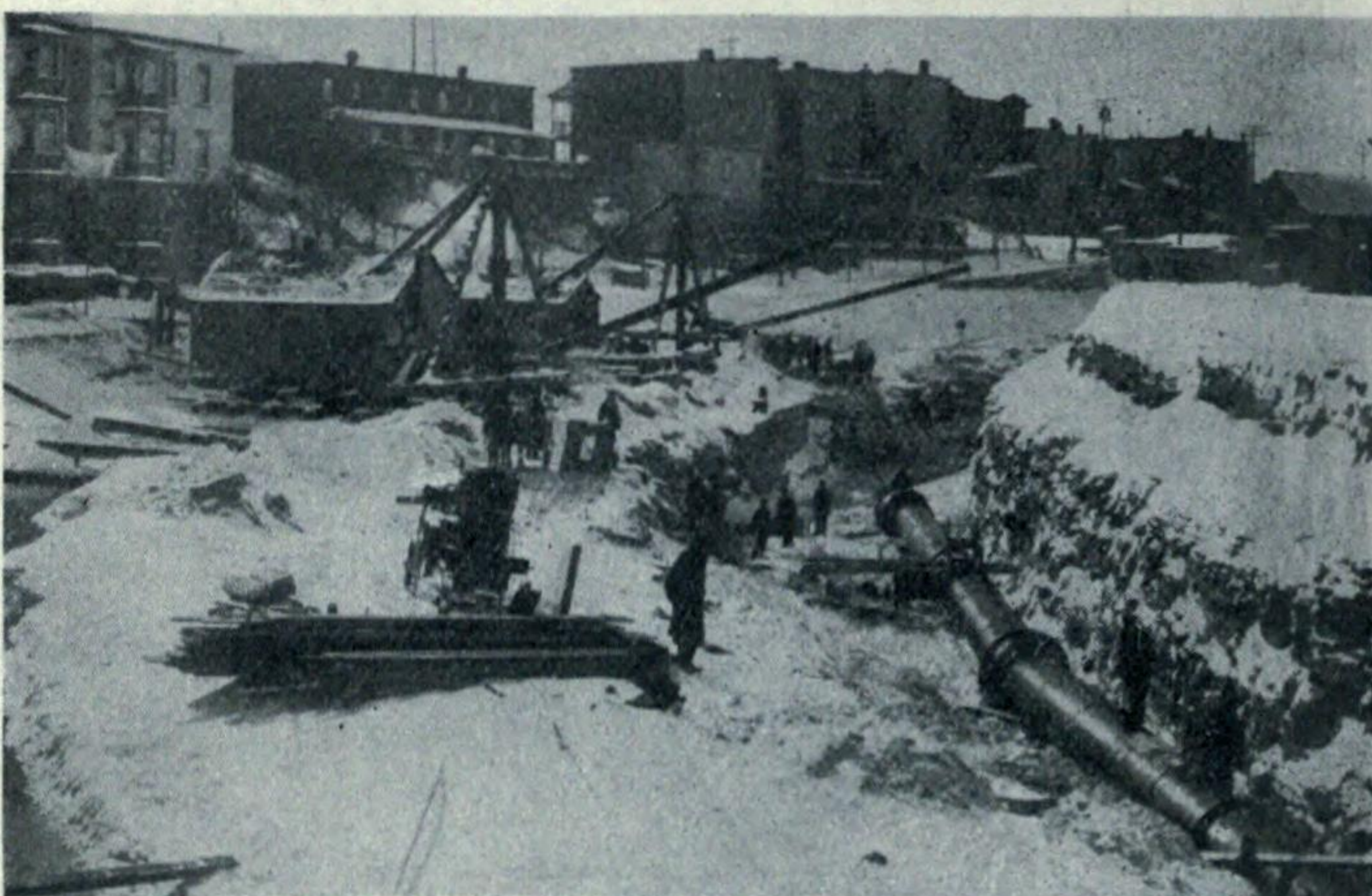
Laying intake pipe. The rock between old and new aqueduct will be removed, forming one large mill pond to overcome anchor ice troubles
