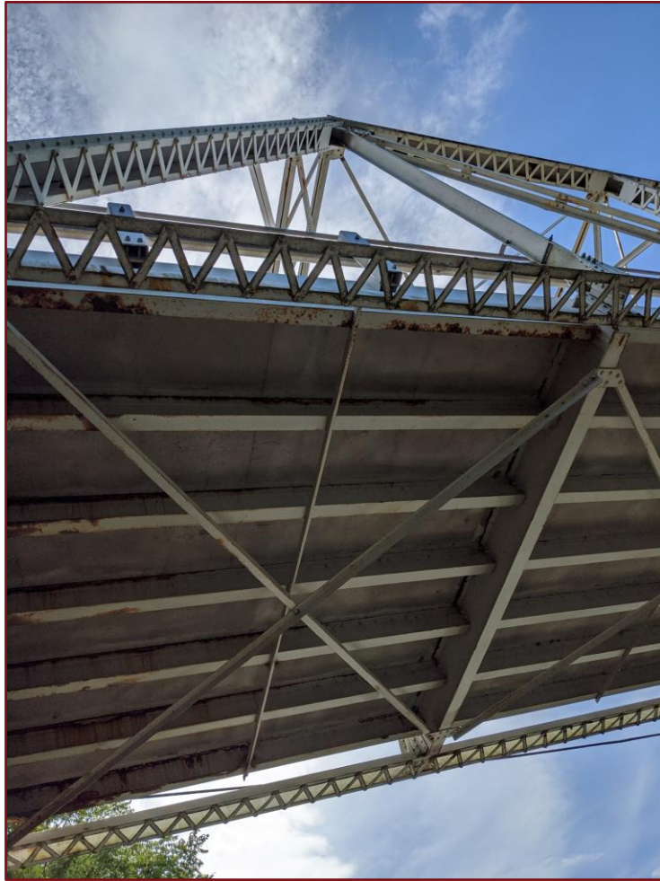
Image 13: Rust Evident on the Underside of the Bridge (Looking West Along the North Bank)
