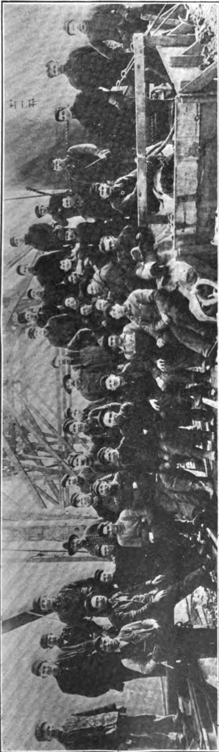
Members of Local No. 3, Pittsburg, Pa., working at Shipperville, Pa., on cantilever bridge for the Lake Shore Railroad. American Contracting Company, contractors.
