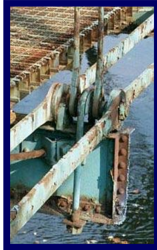
Detail of floor system connecting to truss on the old Utica Bridge while destruction was in progress. photo copyright © 2001 Daniel Alward
