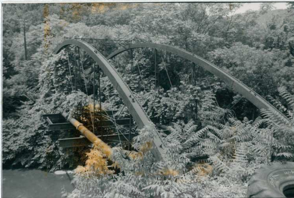
View looking from the east bank across to the west bank of the trolley bridge. Note that the decking has been removed to expose the floor beams.
