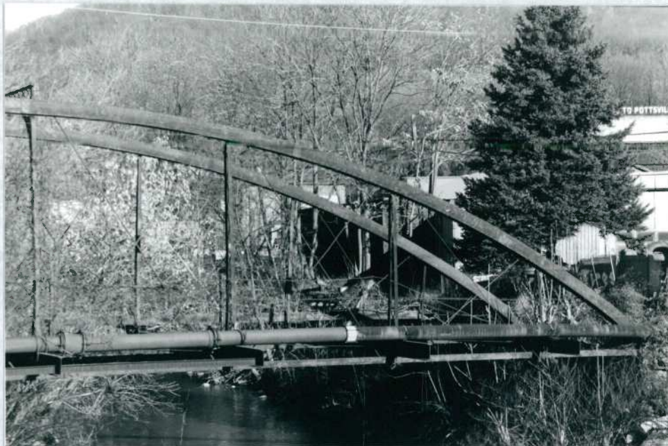
View of bridge, looking north. Note the water pipe which the bridge carries across the Schuylkill River.
