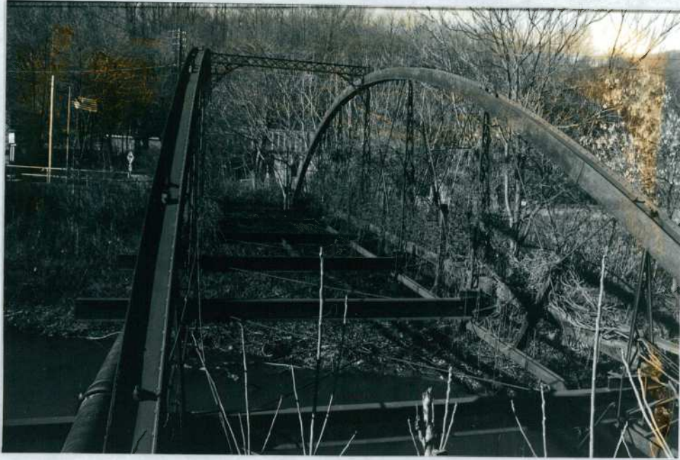
View of bridge, looking west. The bridge has been without decking for several decades. A pedestrian walkway was located on the north side of the bridge.
