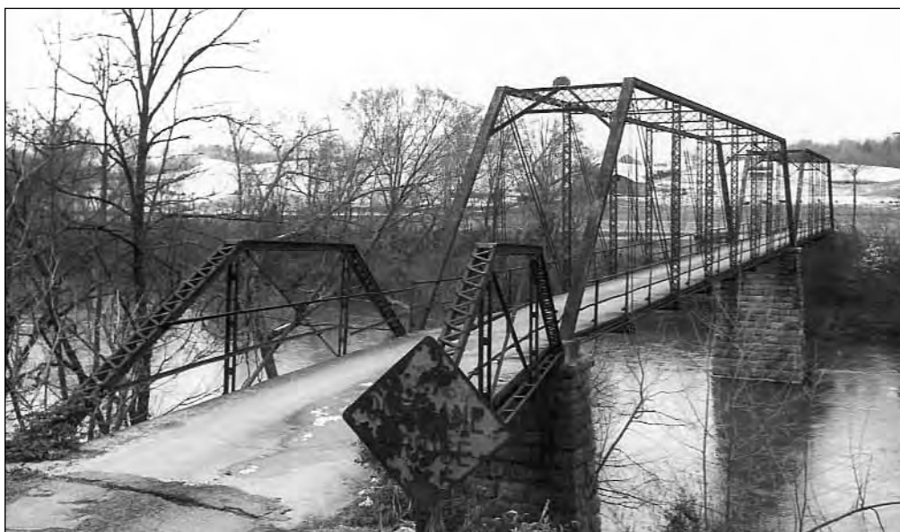
Significant under Criterion C as representative Pratt trusses by the Southern Bridge Company.
