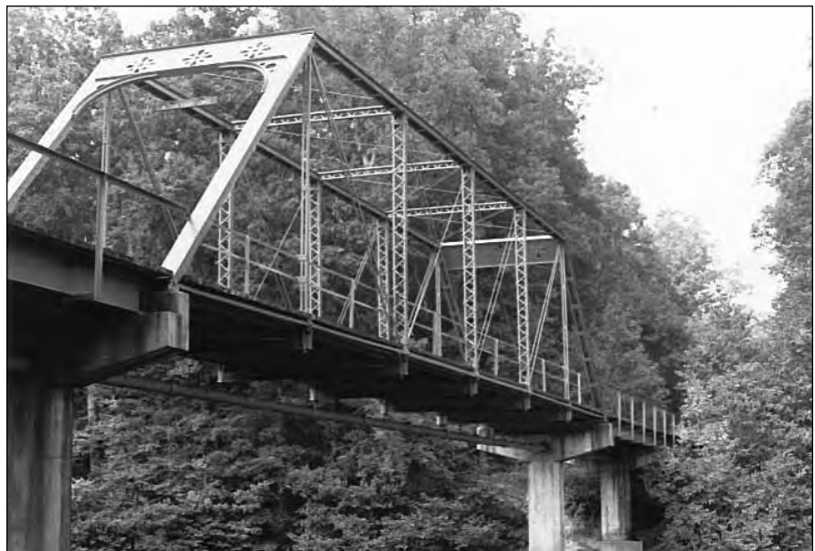
Significant under Criterion C as a representative Pratt truss and as work of the Joliet Bridge Company.
