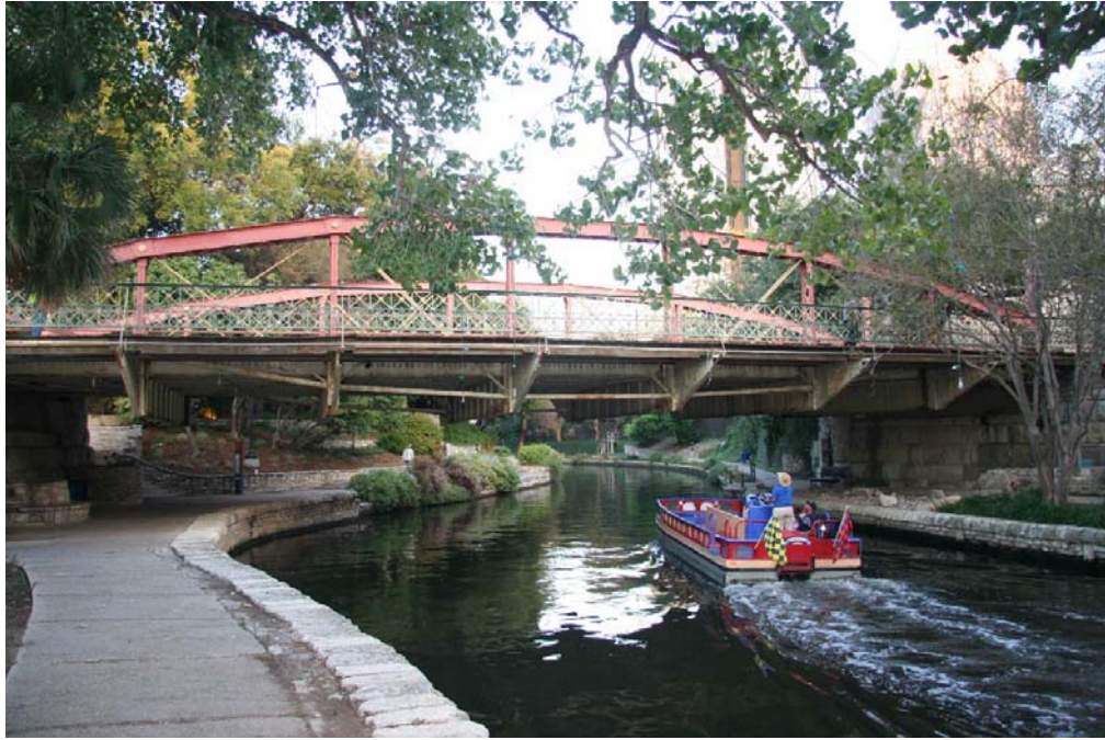
Photo 1: Elevation, facing east, showing the lenticular design of the top and bottom chords that comprise the significant truss type of which this is one of the few known examples in the state
