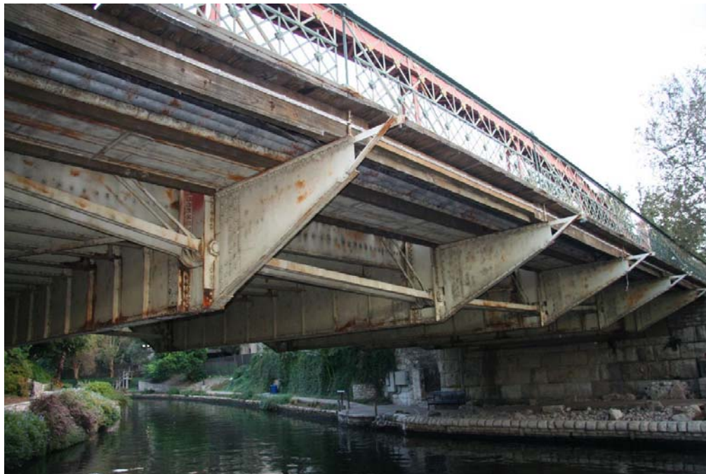
Photo 6: View of underside of truss, facing southeast, including lower chord, built-up floor beams and sidewalk brackets, and stone abutment
