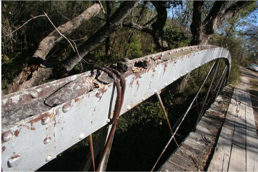
Photo 3: Detail of tubular arch top chord showing tubular construction, threaded-rod connections, and iron castings
