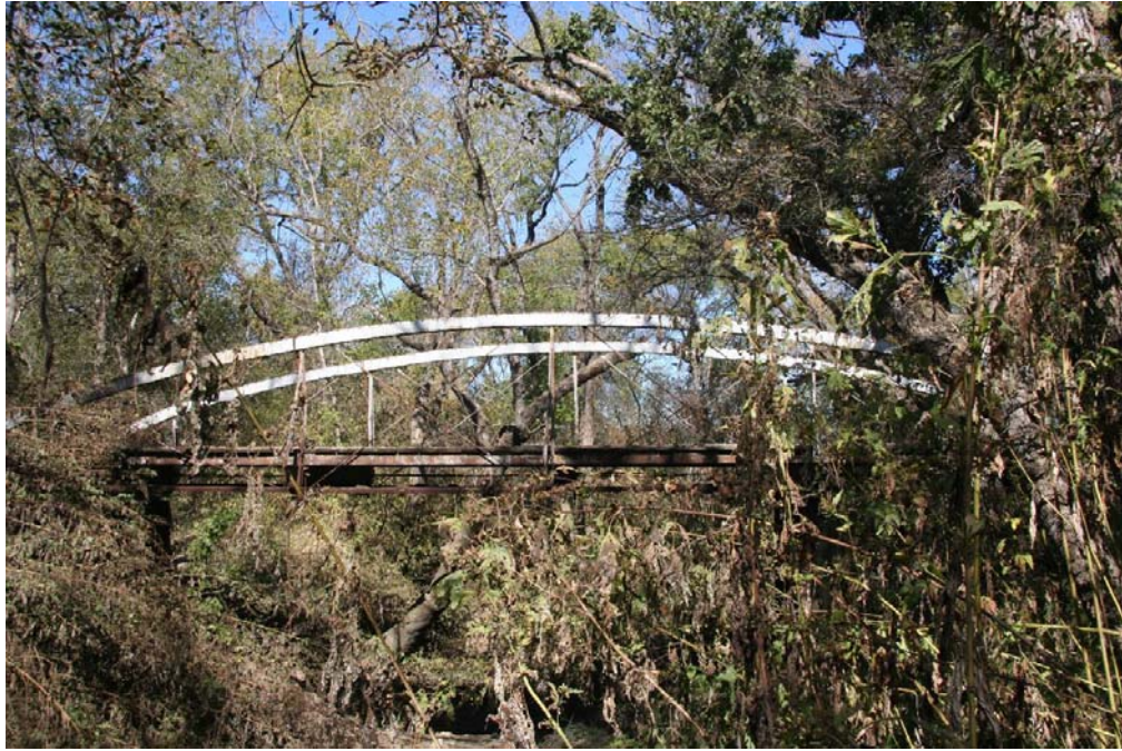
Photo 1: South elevation, facing north, showing the bowstring truss with tubular arch top chord, a rare survivor of a once-common type
