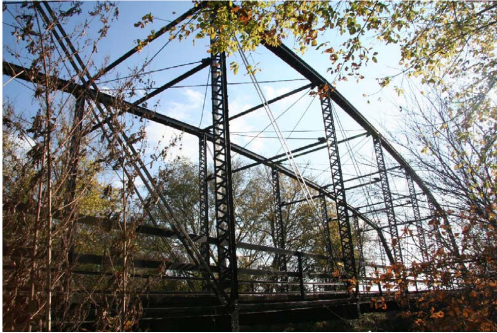
Photo 1: West elevation of the one-span Parker through truss bridge, a rare survivor of a once common truss type; view facing southeast
