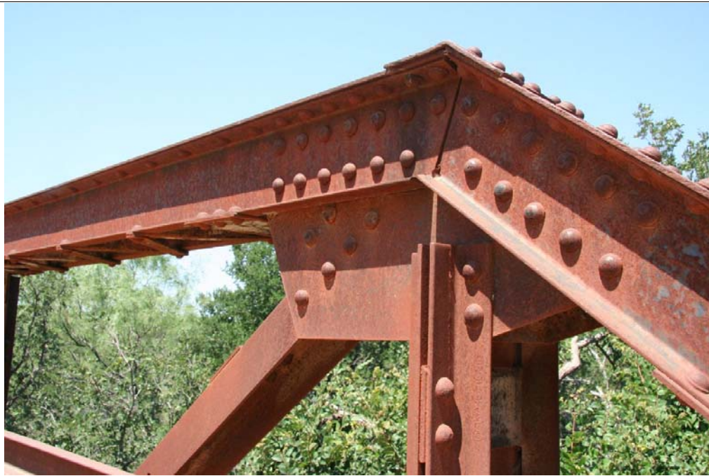
Photo 3: Detail of riveted gusset plate connection at top chord and end diagonal
