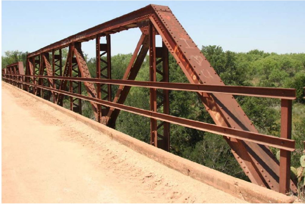
Photo 1: Oblique of truss elevation from deck, facing northwest, showing the Warren pony truss configuration
