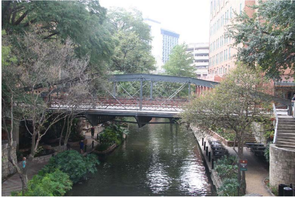
Photo 1: North elevation, facing south, showing the lenticular design of the top and bottom chords that comprise the significant truss type of which this is one of the few known examples in the state
