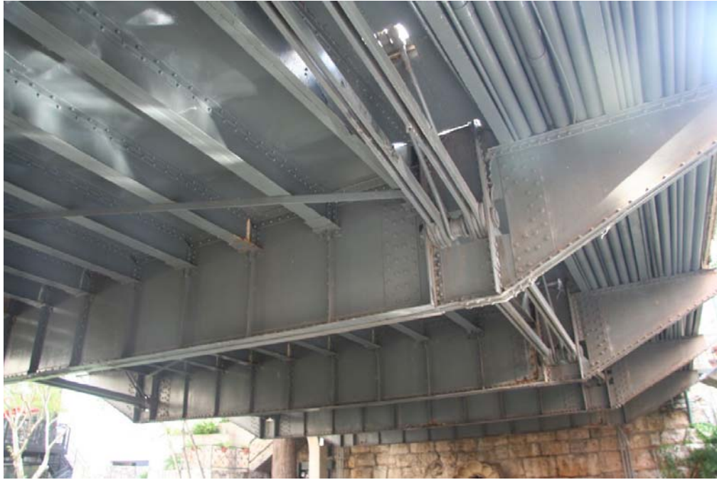
Photo 5: View of underside of truss, facing east, showing built-up floor beams, stringers, and bottom chord with pin connections
