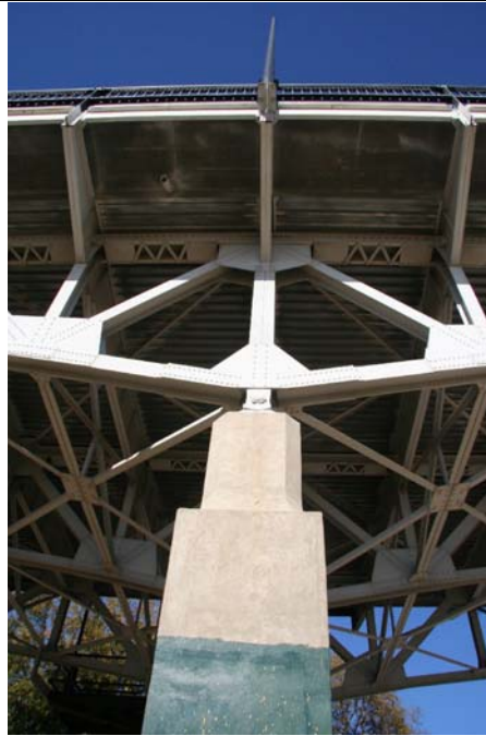
Photo 3: Detail of a bottom chord connection at a pier, showing the continuous design of adjacent spans
