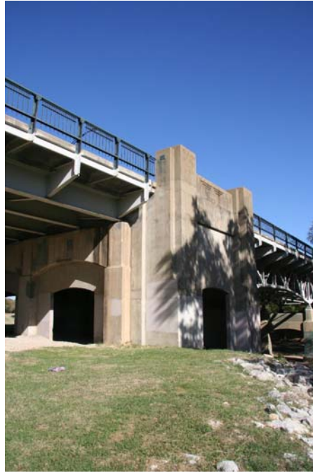
Photo 5: Transitional pier structure between major and minor approach spans, facing northeast, showing architectural detailing
