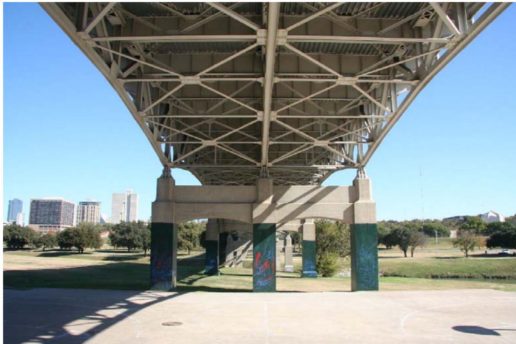
Photo 4: View of underside of truss spans, showing the three lines of trusses
