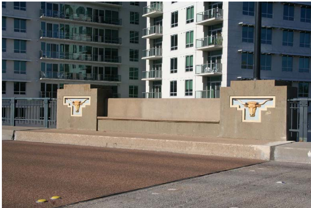
Photo 6: View from deck of ornamental and sculptural treatment of roadway elevation of transitional pier structure
