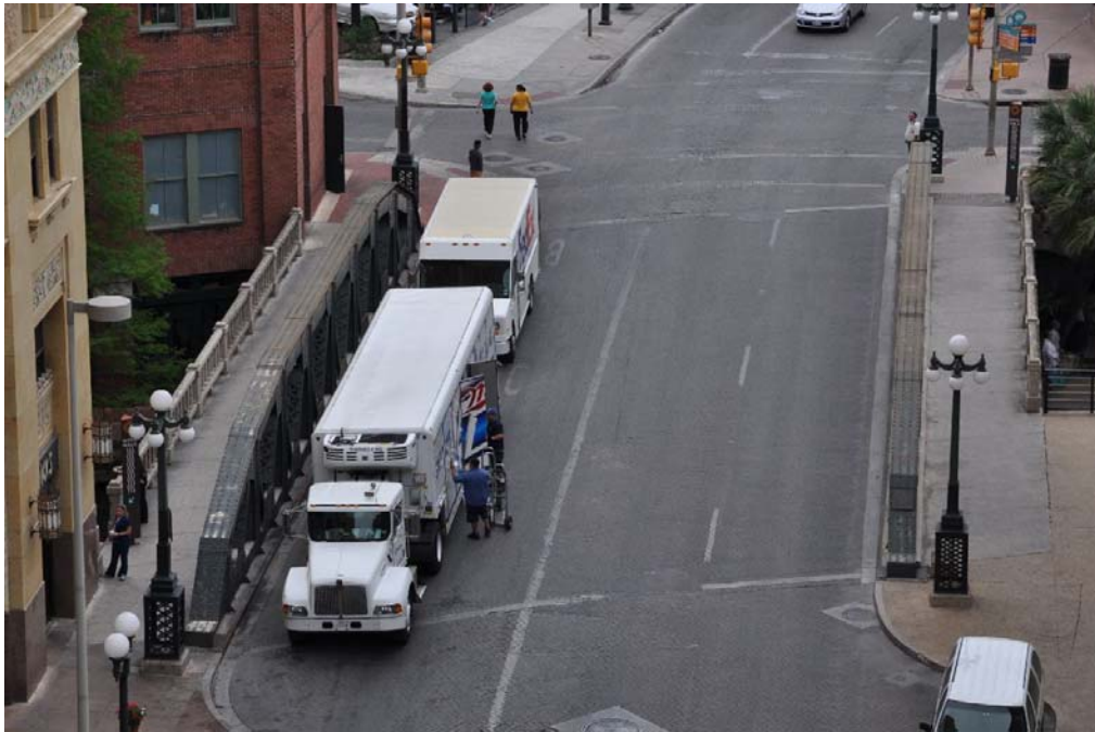
Photo 1: Overview of bridge deck and sidewalks on either side of vehicular lanes; view facing south
