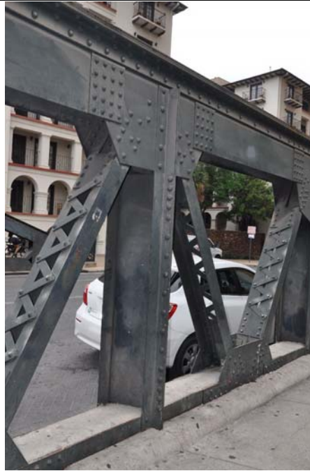
Photo 3: Detail of vertical member with replacement bolts and concrete curb; view facing southeast
