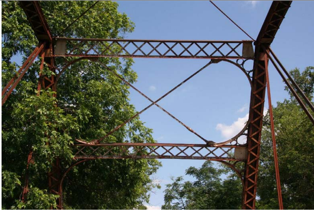
Photo 3: Detail of the decorative portal bracing, which represents the bridge's significance for high artistic value
