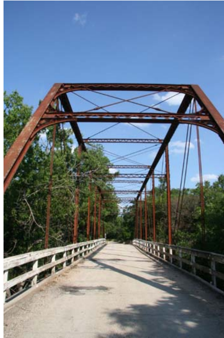
Photo 1: North elevation of the one-span Pratt through truss, a rare survivor of a once-common truss type; view facing southwest
