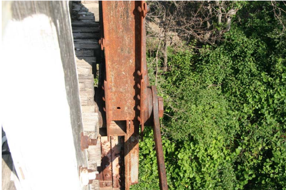
Photo 2: Detail of the primary connection type - the pin connection – that is a significant feature of this bridge due to the date of construction prior to 1900
