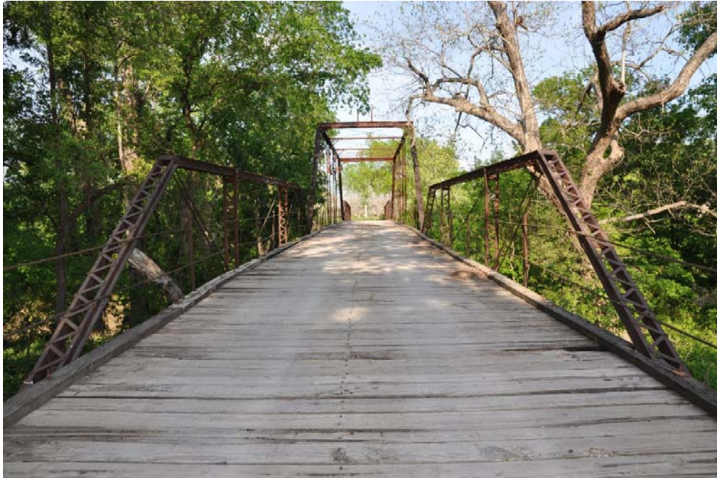
Photo 1: Overview of bridge comprised of a one-span, pin-connected Pratt through truss, which is a rare survivor of a once-common type, one-span Pratt pony truss, and one-span Warren pony truss; view facing northeast
