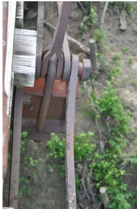
Photo 2: Detail of primary pin connection and the U-bolt at the bottom chord
