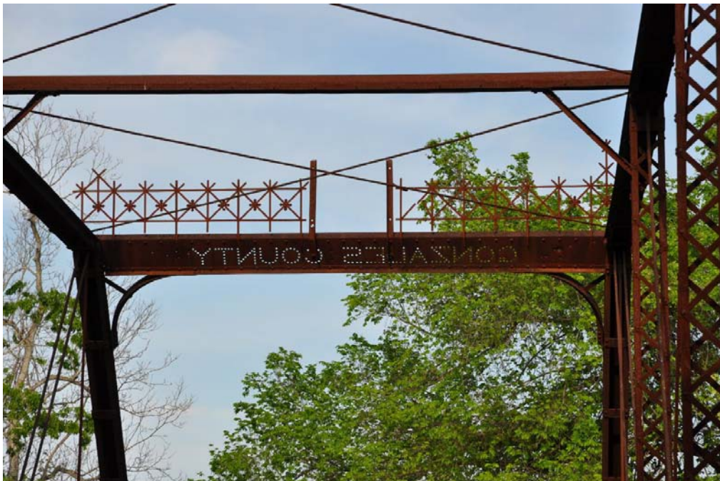
Photo 6: Detail of decorative portal, cresting, and knee bracing on the Pratt through truss main span
