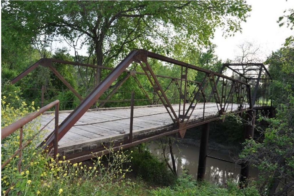
Photo 5: Elevation of bridge, primarily the Warren pony truss span; view facing southwest
