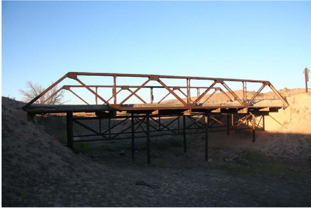
Photo 1: South elevation, facing north, showing the design of the Warren pony truss with parallel chord
