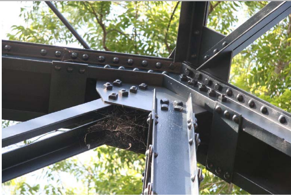
Photo 3: Detail of primary structural connection at top chord, end post, and portal
