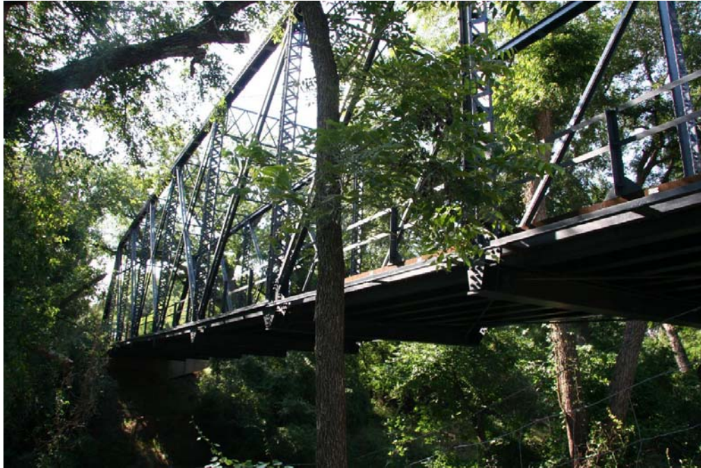
Photo 1: Elevation of the one-span Pratt through truss; a rare survivor of a once-common truss type; view facing southeast
