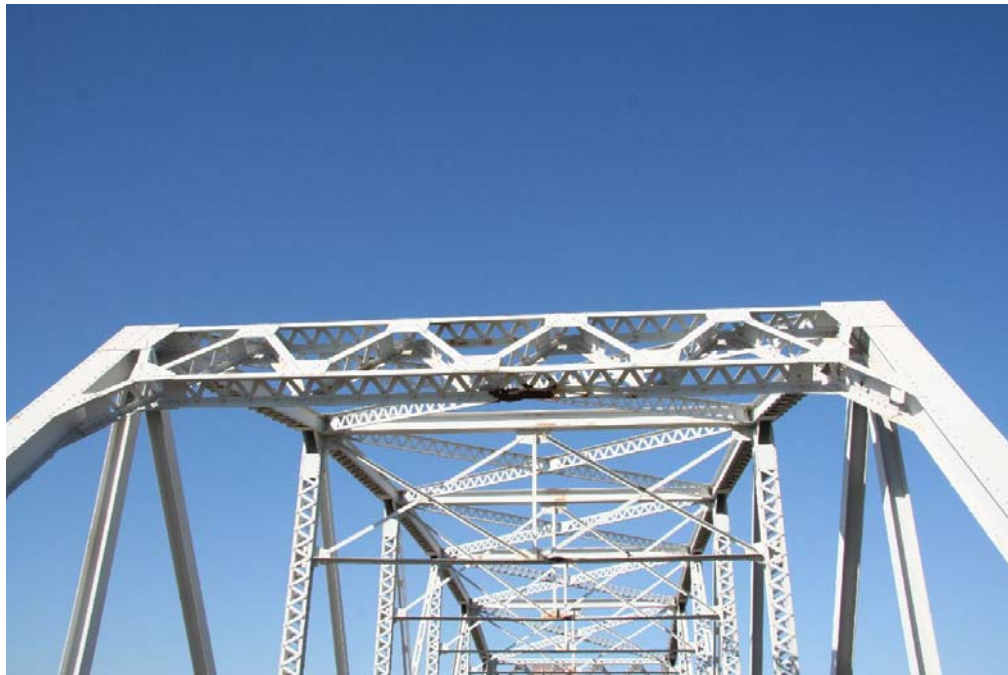
Photo 4: Detail of impact damage on portal and sway bracing; view facing north
