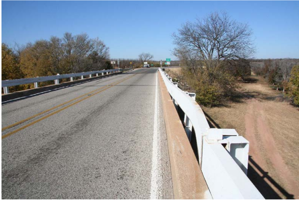
Photo 5: Detail of impact damage on approach span railing; view facing north
