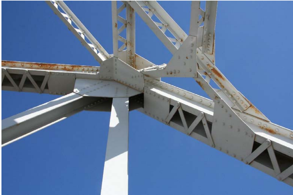
Photo 2: Detail of primary truss connection type at endpost and top chord of south truss span; view facing east
