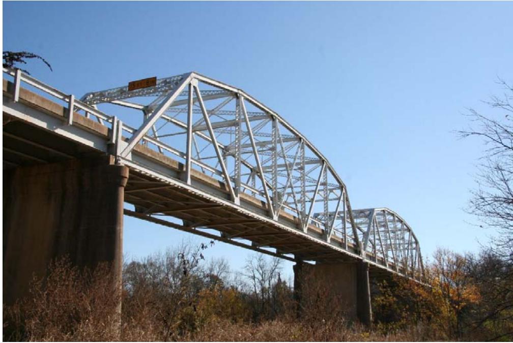
Photo 1: West elevation of structure comprised of two Parker through trusses, a rare survivor of a once-common truss type; view facing southeast
