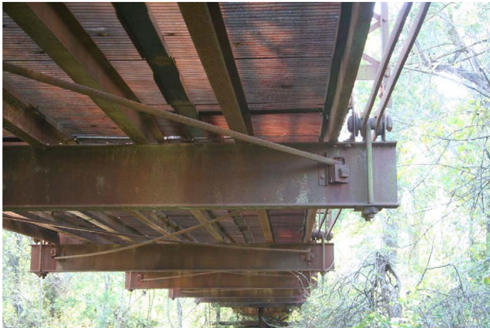
Photo 4: Detail of primary connection at the bottom chord, including the U-bolt connection at the floor beam
