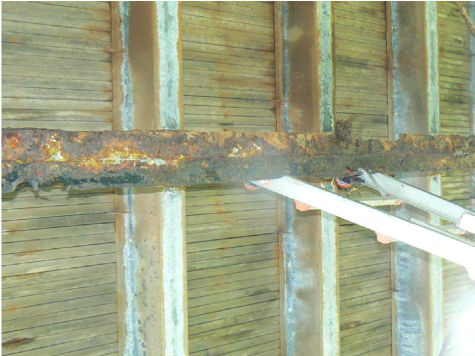
Severe rusting and section loss in deck supports.
