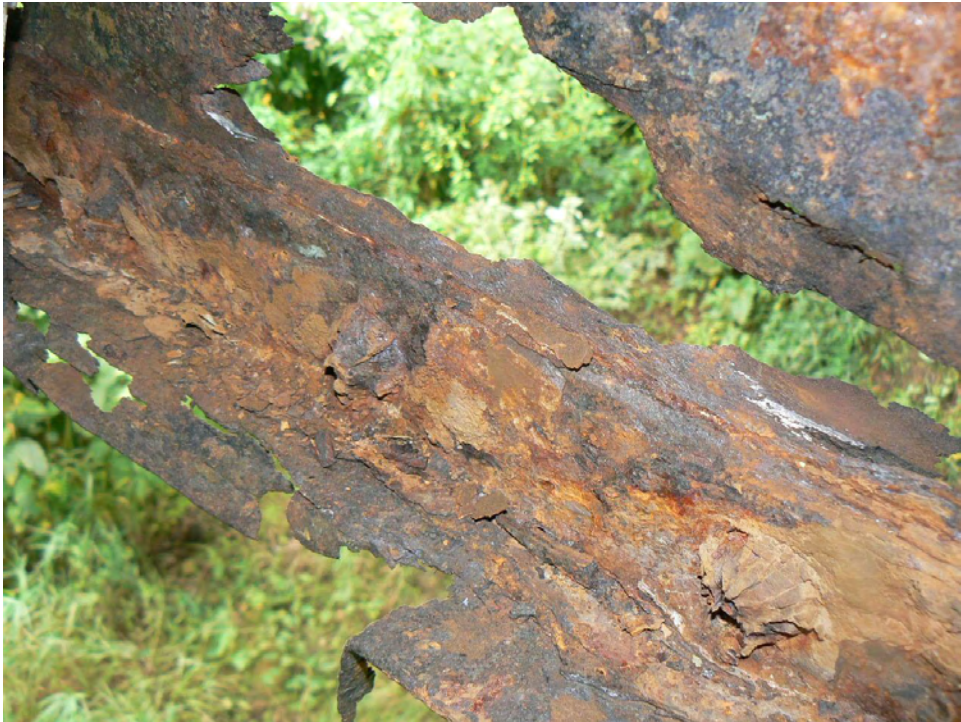
Severe rusting and section loss of supports.
