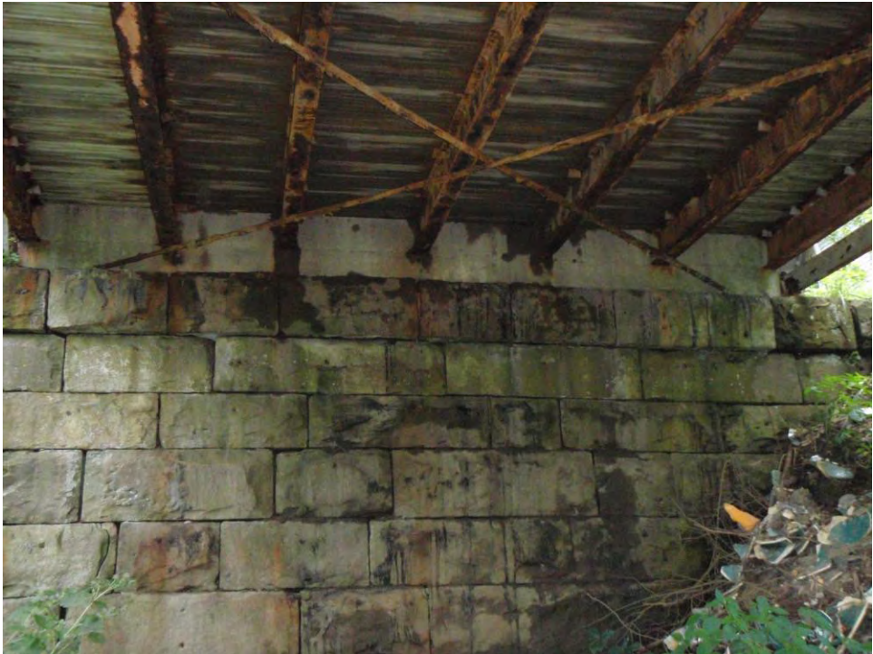
Rusting and deterioration of floor beams and supports.
