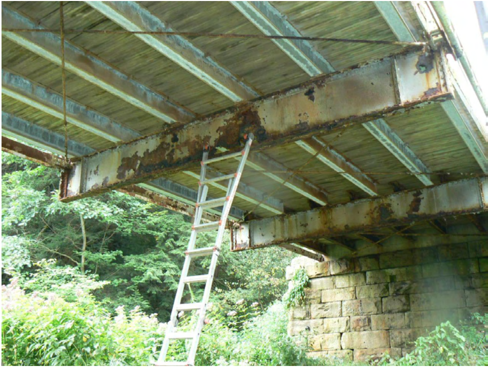
Rusting and section loss in floor beams.
