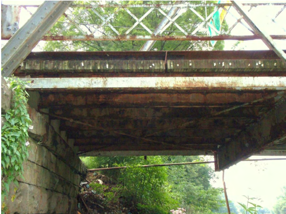
Rusting and deterioration of Truss members and floor beams/supports.
