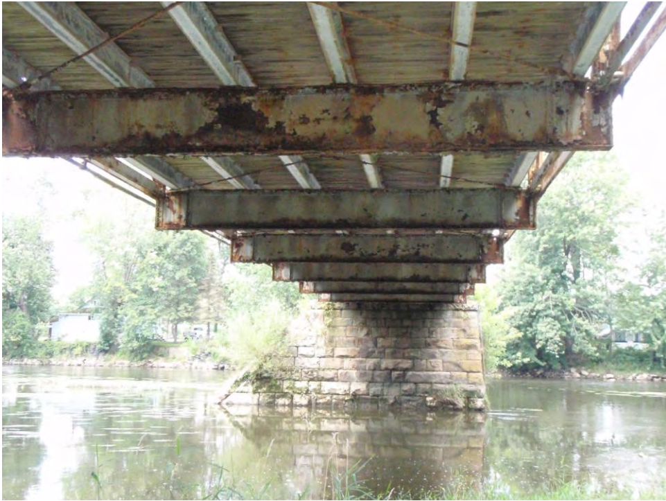
Deterioration and rusting of superstructure.
