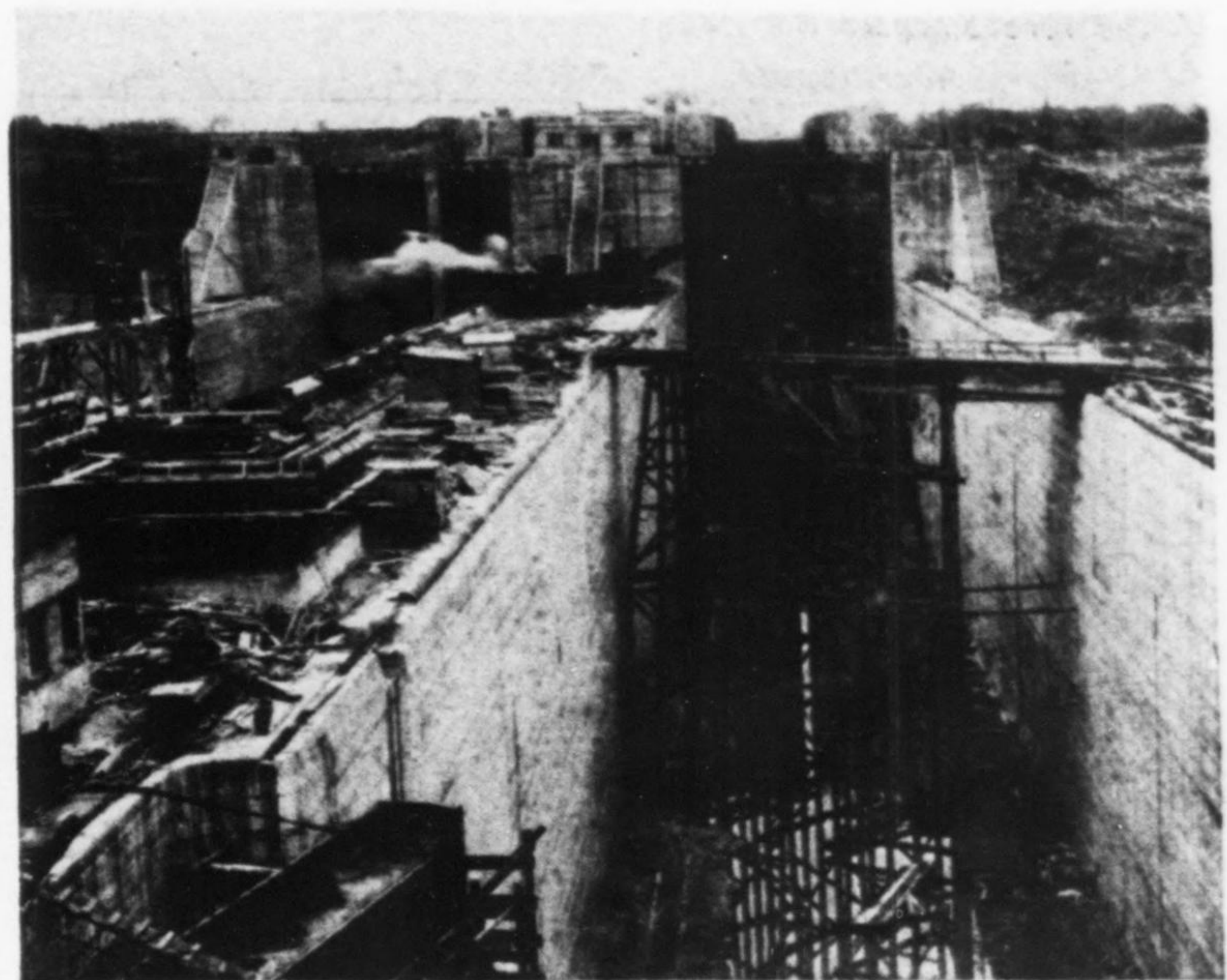
FIG. 6—TWIN FLIGHT LOCKS AT THOROLD Looking up the flight of three twin locks at Thorold from the C. N. Ry. bridge. The lock chambers are 80 ft. wide and 82 ft. deep. The three locks give a total lift of 139.5 ft. (The C. N. Ry. bridge shown above the lower of these locks on the cover of this issue has been replaced by a rolling lift bridge.)
