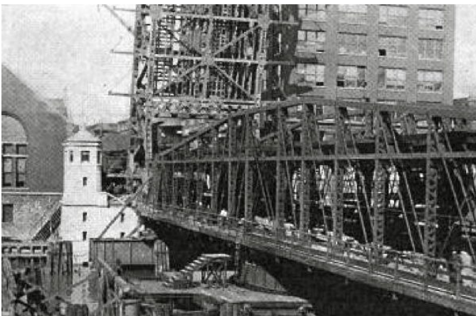
View of the north leaf of the Wells St. bridge under construction with the existing swing bridge in place - 1922. (Photograph from "Engineering World," Volume 20, June - January, 1922 - as digitized by Google books)
